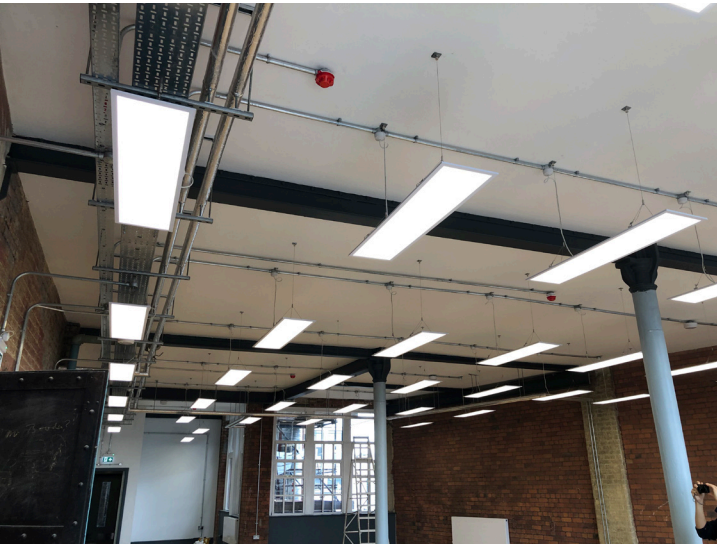
Image showing existing cable trays and lighting to the upper floors at 86 Princess Street. Similarly, the new lighting is to be fixed to the underside of trays or to the plastered soffits.
