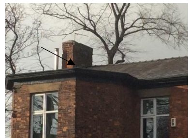
B2; Lifted ridge roof slate
