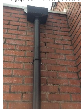
B1; gaps in the mortar
