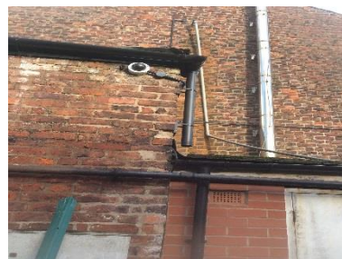
B2a; Lifted roof felt
