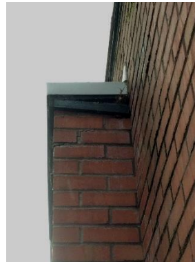
B1; gap behind bargeboard
