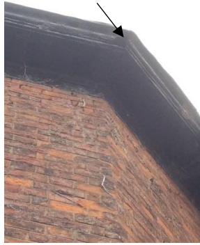
B2; Large hole in soffit box
