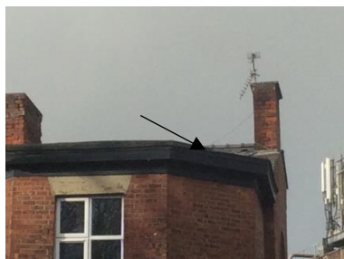
B2; Slipped roof slate
