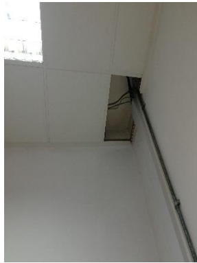
B2; Missing tile revealing roof
