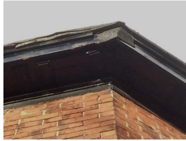
B2; Lifted felt above soffit box
