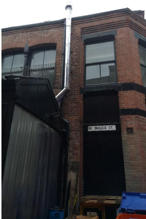
Figure 4.3: View of similar extraction system on Back Bridge Street.
