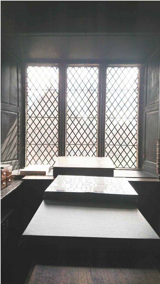
⑯ Window soffit paneling has been over-boarded with 2-3 mm hardboard but frame remains intact.
