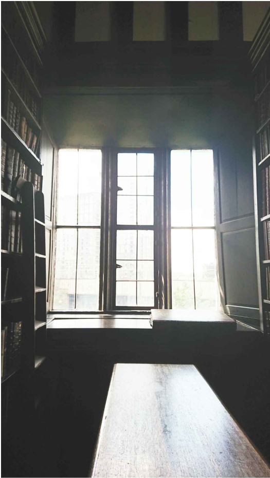
⑨ Window soffit paneling has been over-boarded with 2-3 mm hardboard but frame remains intact.
