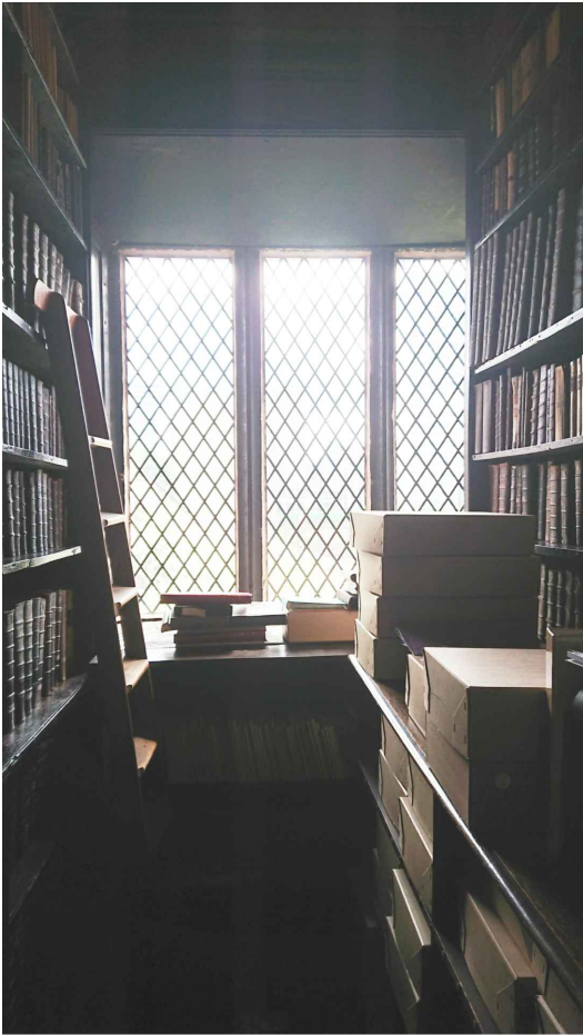
⑬ Window soffit paneling has been over-boarded with 2-3 mm hardboard - paneling and frame are presumed to have been removed.
