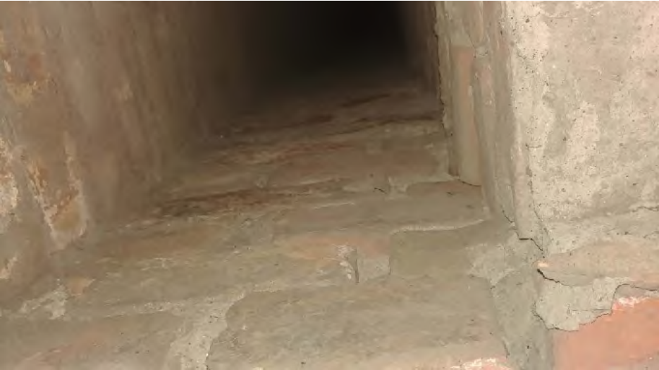
Voids not Visible above an Opening
