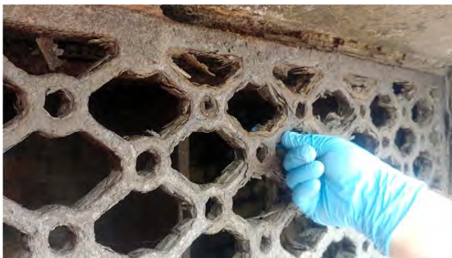
Plate T4: The decorative grilles were also very badly corroded.
