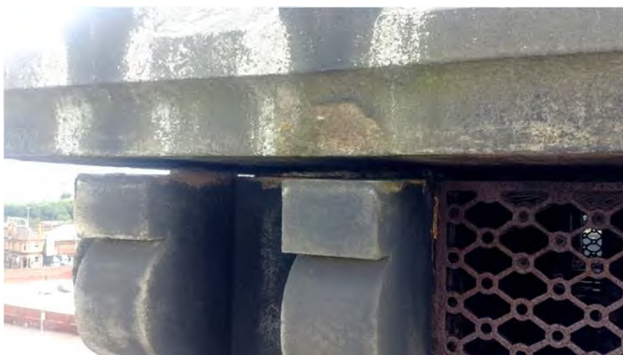
Plate T6: Displaced supporting corbels.
