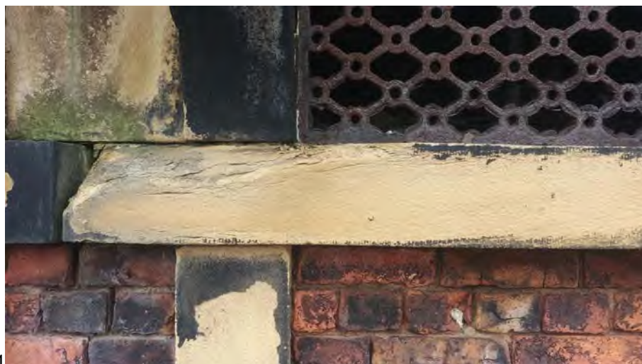
Plate T5: Spalled top corner of a stone sill.
