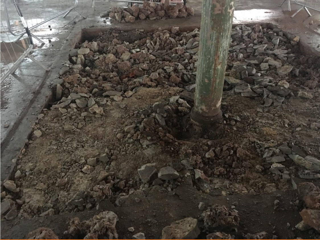
PLATE 3 MADE GROUND IN BASE OF LIFT SHAFT
