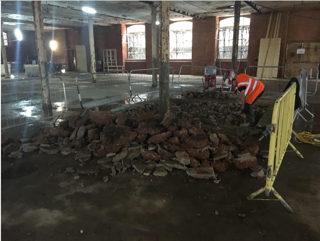
PLATE 1 BROKEN CONCRETE IN AREA OF LIFT SHAFT
