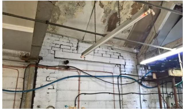
Plate 23: Gaps in Brickwork
