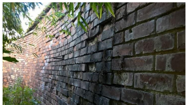
Plate 5: Missing/Degraded Brickwork on the Western Side of the Building
