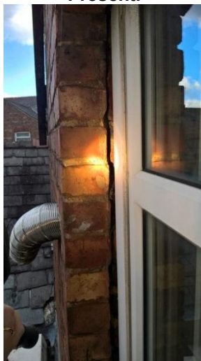
Plate 14: Gaps Around the Central Office Window (Southern Elevation).
