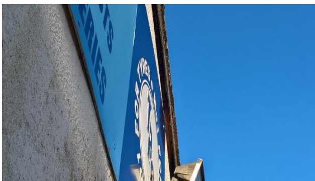
Plate 41: Gaps Behind Barge Board Eastern Gable End.
