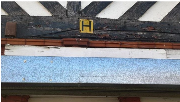
Plate 8: Raised Brickwork Above Shutter Box.
