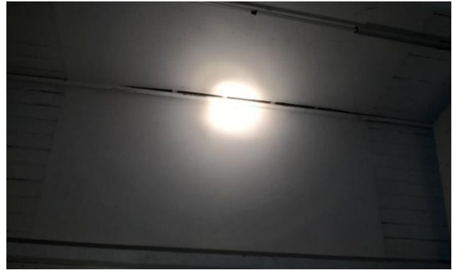
Plate 29: Gaps Recorded at the Roof Apex.
