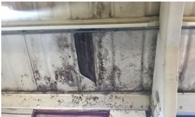
Plate 43: Concrete Composite Coating Peeling Away from the Corrugated Metal Roof
