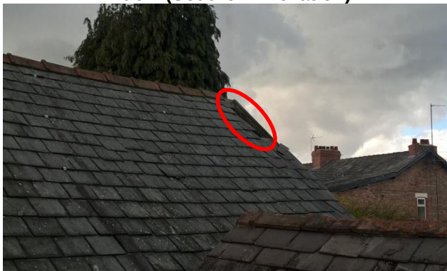
Plate 16: Hole in North-west Corner of Sewing Workshop Roof.
