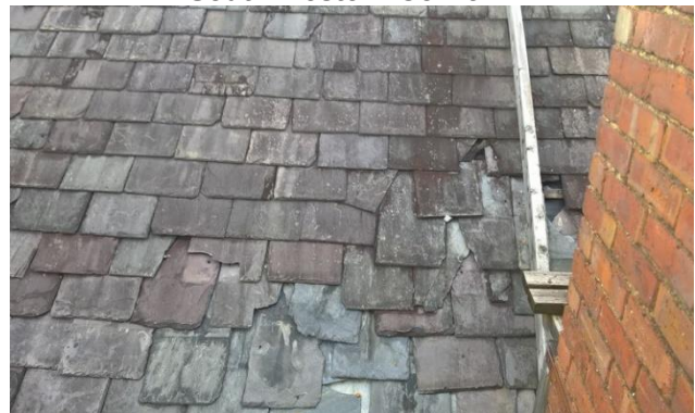
Plate 17: Slipped Slate Tiles on Eastern Elevation of Western-most Roof Section.
