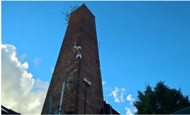
Plate 11: The Tall Chimney with Crumbling Brickwork to the North.
