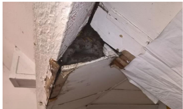
Plate 32: The Exposed Insulation to the South-east of the Sewing Room.
