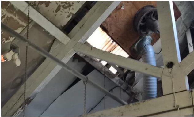
Plate 22: Lifted Ceiling Boards and Plastic Sheeting.
