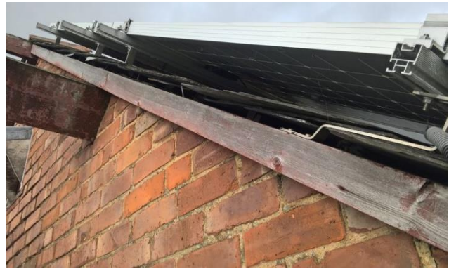
Plate 13: Gaps at the Eaves of Central Office Section
