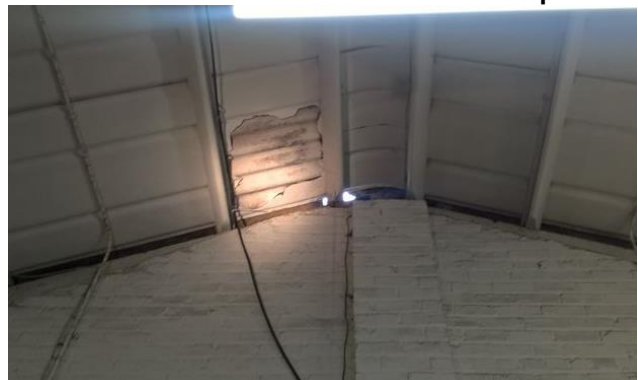
Plate 44: Peeling Concrete Composite Coating and Gaps at the Western Gable End
