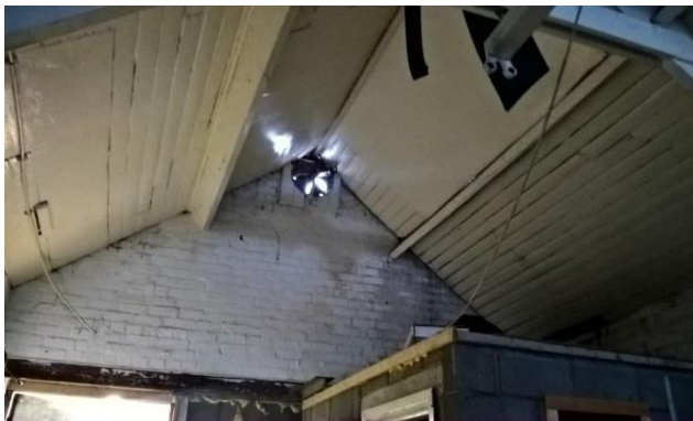
Plate 30: Old Fan Unit to the South with Breezeblock Structure below.
