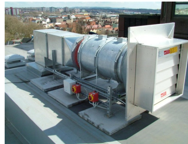
Typical duty and standby smoke extract fan
