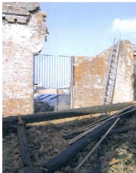
Figure 42 – An unknown area of collapse in October 2005.
