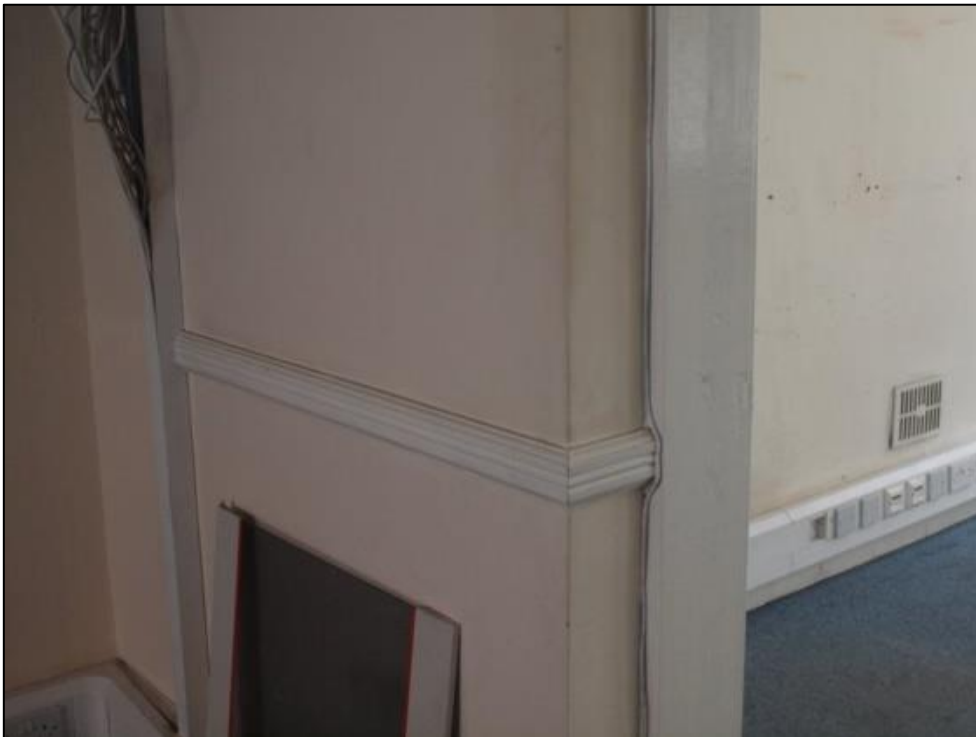
Plate 39: Detail of modern dado rail, cut by trunking
