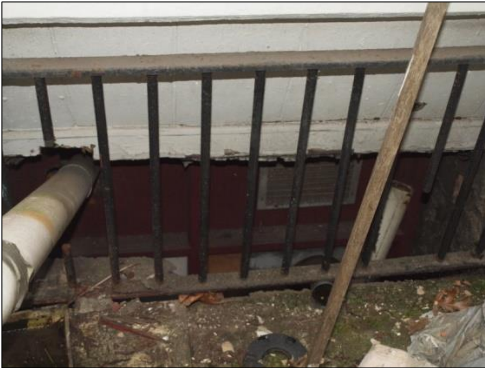
Plate 10: Blocked light well below bay window
