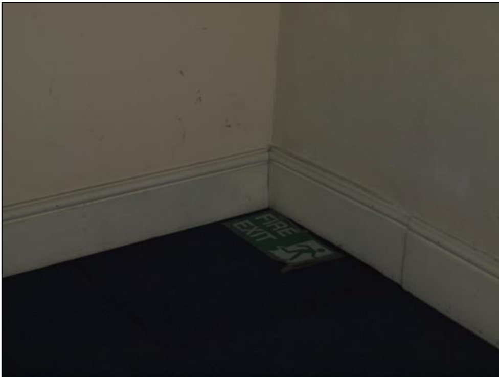
Plate 53: Skirting on top landing
