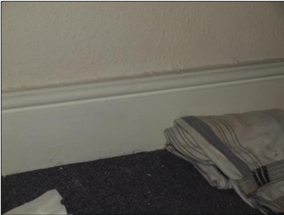
Plate 26: Detail of modern skirting in northwest extension
