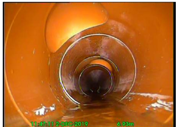
Photo: 19_5A 7.1m, Connection other than junction, at 11 o'clock, diameter 100mm
