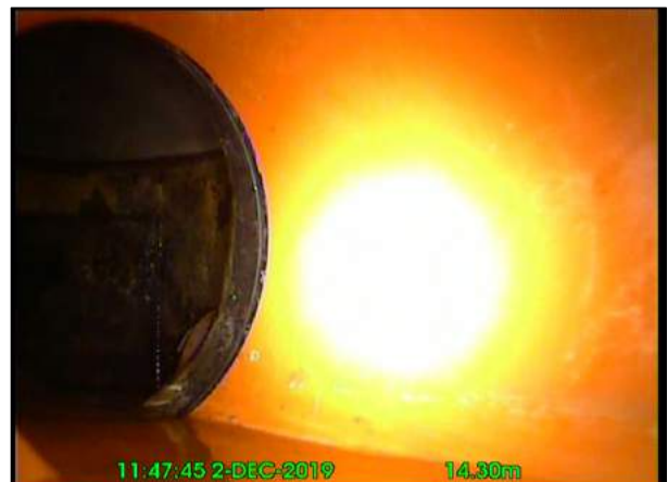
Photo: 19_9A 14.5m, Line deviates left
