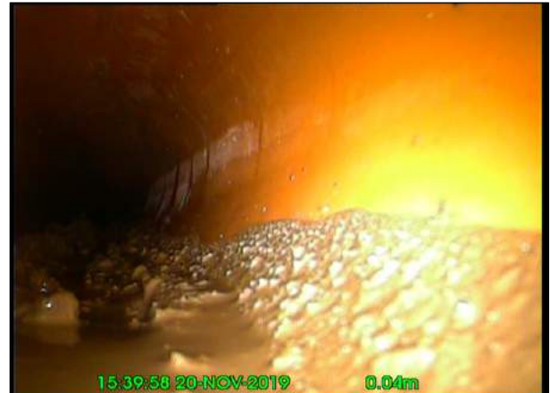
Photo: 7_3A 0m, Settled deposits, fine, 10% cross-sectional area loss, Start
