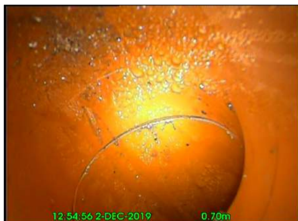
Photo: 21_3A 0.9m, Line deviates down
