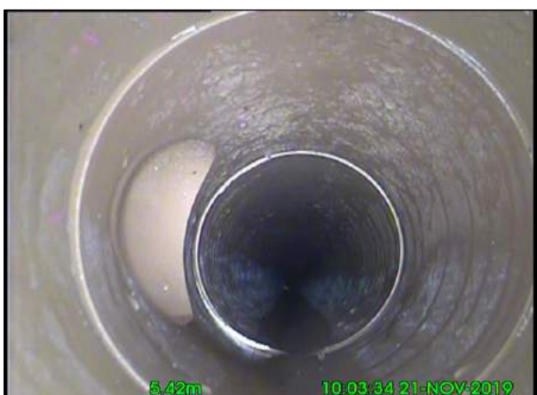
Photo: 15_5A 5.7m, Connection other than junction, at 9 o'clock, diameter 100mm
