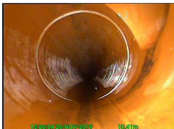
Photo: 4_5A 10.6m, Connection other than junction, at 2 o'clock, diameter 100mm
