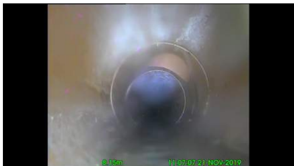
Photo: 13_8A 8.5m, Connection other than junction, at 1 o'clock, diameter 100mm
