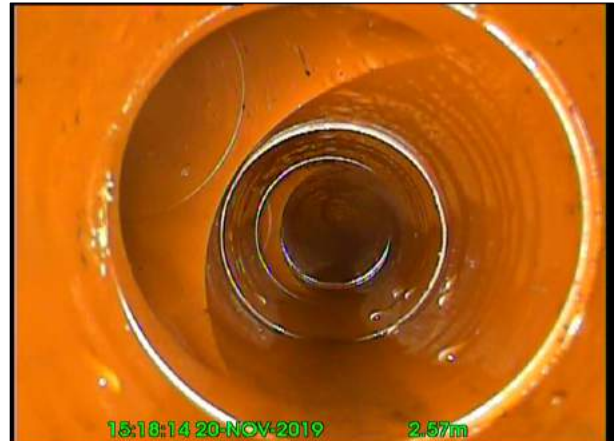
Photo: 5_3A 2.9m, Connection other than junction, at 10 o'clock, diameter 150mm
