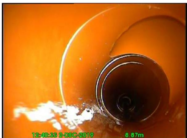
Photo: 20_6A 9.2m, Connection other than junction, at 1 o'clock, diameter 150mm
