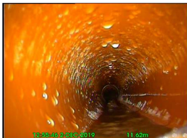
Photo: 21_7A 11.62m, Turbid water level, 10% of the vertical dimension
