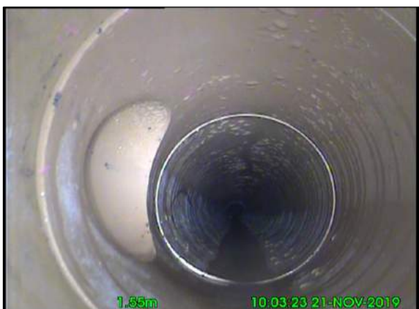
Photo: 15_3A 1.8m, Connection other than junction, at 9 o'clock, diameter 100mm
