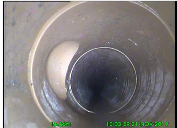
Photo: 15_8A 17m, Connection other than junction, at 9 o'clock, diameter 100mm
