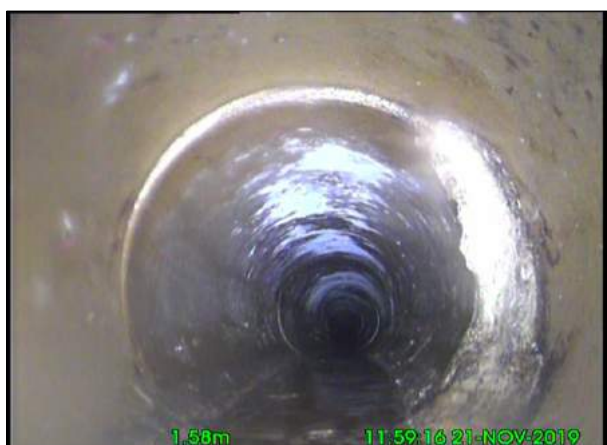
Photo: 11_3A 1.9m, Attached deposits, encrustation at joint, from 1 to 5 o'clock, 10% cross-sectional area loss
