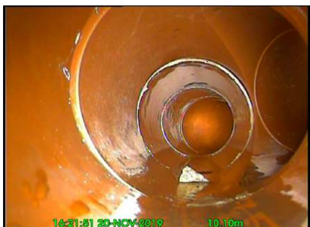
Photo: 3_4A 10.3m, Connection other than junction, at 3 o'clock, diameter 150mm
