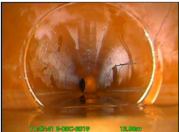
Photo: 19_8A 13.1m, Joint displaced, medium
