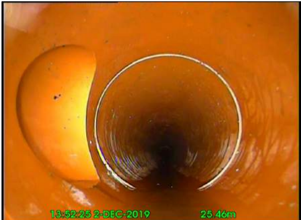
Photo: 24_14A 25.7m, Connection other than junction, at 9 o'clock, diameter 100mm
