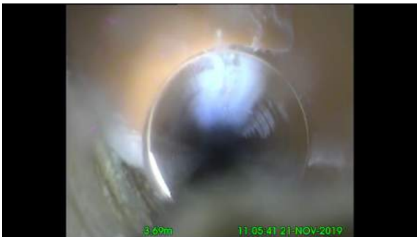
Photo: 13_4A 3.8m, Connection other than junction, at 11 o'clock, diameter 100mm
