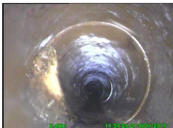
Photo: 11_5A 3.7m, Attached deposits, encrustation at joint, from 6 to 10 o'clock, 15% cross-sectional area loss
