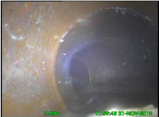
Photo: 11_9A 7.8m, Line deviates left
