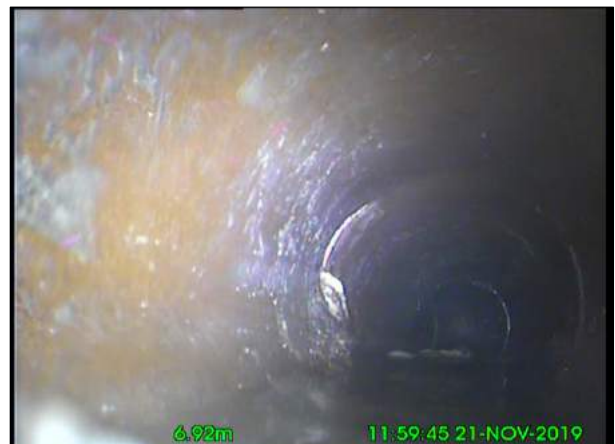
Photo: 11_9A 7.3m, Attached deposits, encrustation at joint, from 6 to 9 o'clock, 15% cross-sectional area loss
