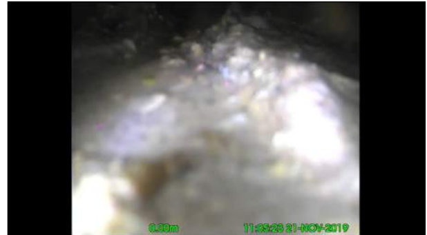
Photo: 13_3A 0m, Settled deposits, fine, 15% cross-sectional area loss, Start
