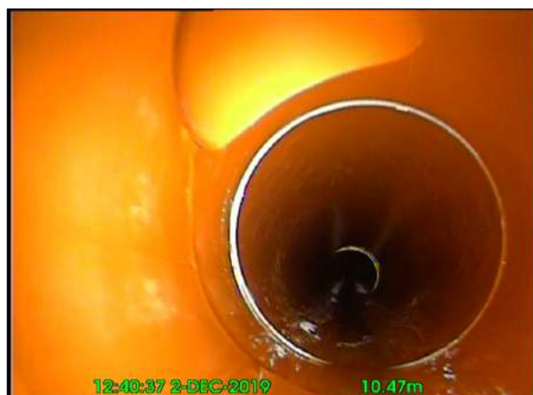
Photo: 20_7A 10.6m, Connection other than junction, at 11 o'clock, diameter 100mm
