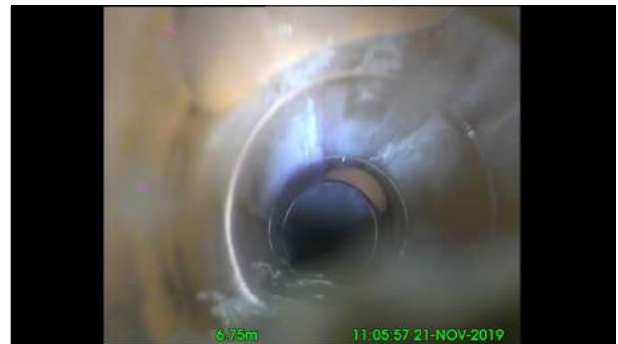
Photo: 13_5A 6.9m, Connection other than junction, at 11 o'clock, diameter 100mm
