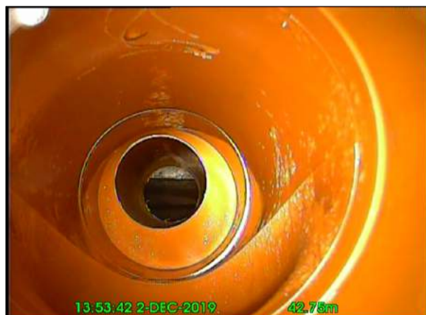
Photo: 24_25A 42.8m, Survey abandoned Remarks: Unable to pass drop shaft
