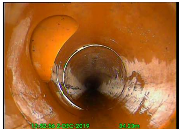
Photo: 24_17A 34.5m, Connection other than junction, at 10 o'clock, diameter 100mm
