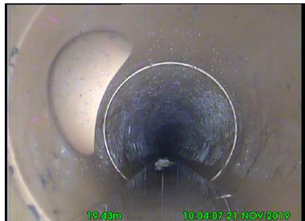
Photo: 15_10A 19.6m, Connection other than junction, at 9 o'clock, diameter 100mm
