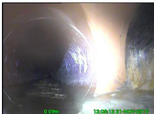
Photo: 12_3A 0.1m, Connection other than junction, at 3 o'clock, diameter 150mm
