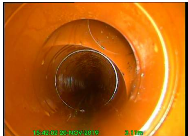
Photo: 8_5A 3.3m, Connection other than junction, at 1 o'clock, diameter 100mm
