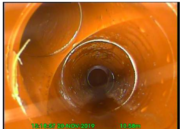
Photo: 5_5A 10.7m, Connection other than junction, at 10 o'clock, diameter 150mm
