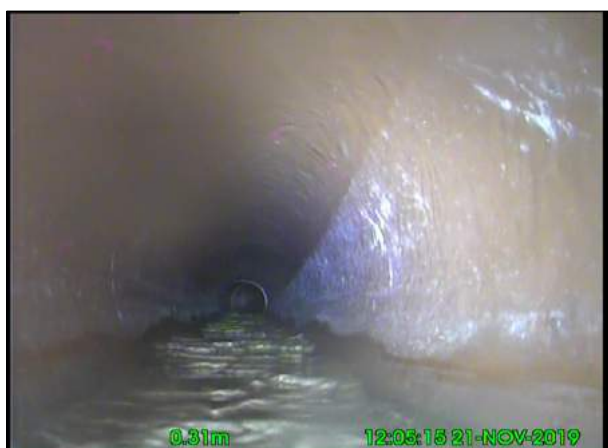
Photo: 12_4A 0.4m, Settled deposits, fine, 15% cross-sectional area loss, Start
