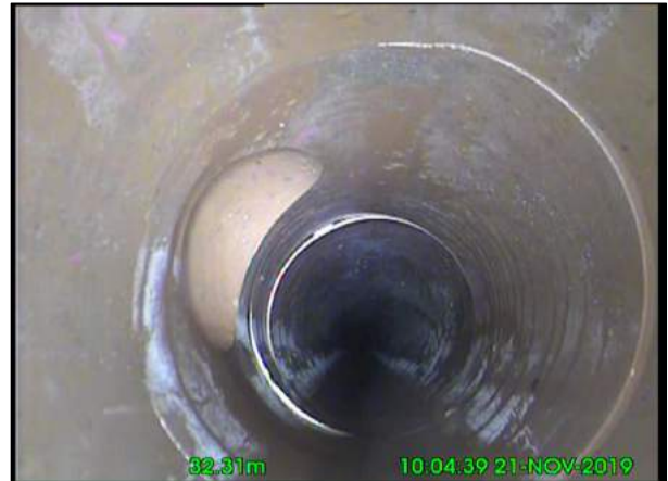
Photo: 15_17A 32.5m, Connection other than junction, at 10 o'clock, diameter 100mm
