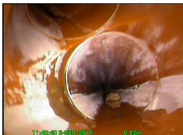
Photo: 23_5A 1m, Connection other than junction, at 11 o'clock, diameter 150mm
