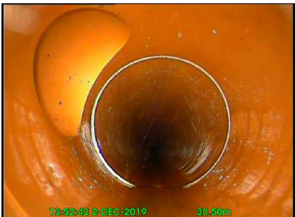
Photo: 24_16A 30.7m, Connection other than junction, at 10 o'clock, diameter 100mm
