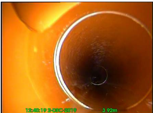
Photo: 20_4A 4m, Connection other than junction, at 11 o'clock, diameter 100mm
