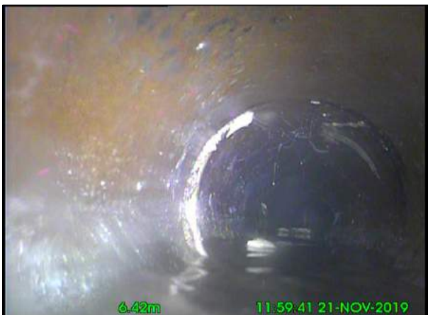
Photo: 11_8A 6.6m, Joint displaced, medium
