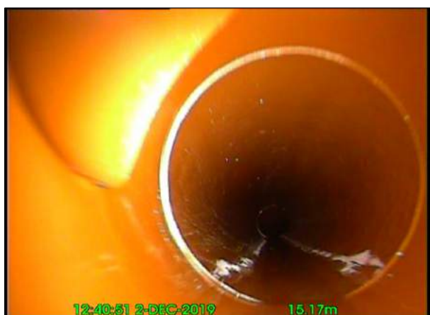
Photo: 20_8A 15.4m, Connection other than junction, at 10 o'clock, diameter 100mm
