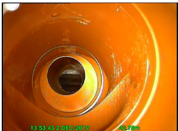
Photo: 24_24A 42.8m, Connection other than junction, at 6 o'clock, diameter 100mm
