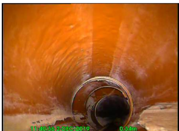
Photo: 23_4A 0.3m, Attached deposits, encrustation, from 3 to 4 o'clock, 10% cross-sectional area loss
