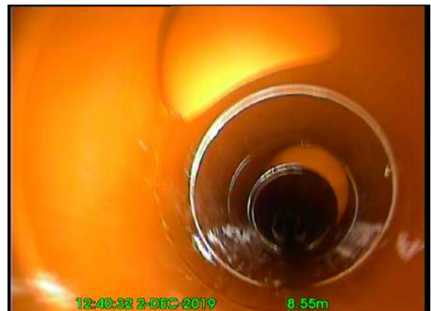
Photo: 20_5A 8.8m, Connection other than junction, at 11 o'clock, diameter 100mm
