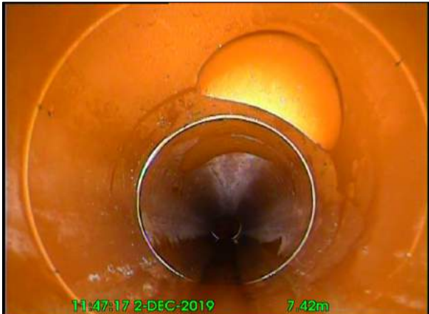
Photo: 19_6A 7.6m, Connection other than junction, at 1 o'clock, diameter 100mm
