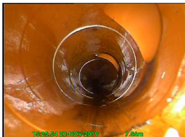
Photo: 4_3A 7.8m, Connection other than junction, at 2 o'clock, diameter 100mm
