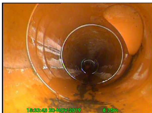
Photo: 6_6A 9m, Connection other than junction, at 2 o'clock, diameter 100mm
