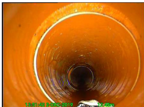
Photo: 24_7A 12.7m, Joint displaced, large
