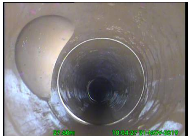
Photo: 15_15A 27.8m, Connection other than junction, at 10 o'clock, diameter 100mm
