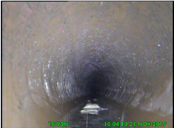
Photo: 15_11A 19.95m, Settled deposits, fine, 10% cross-sectional area loss, Start
