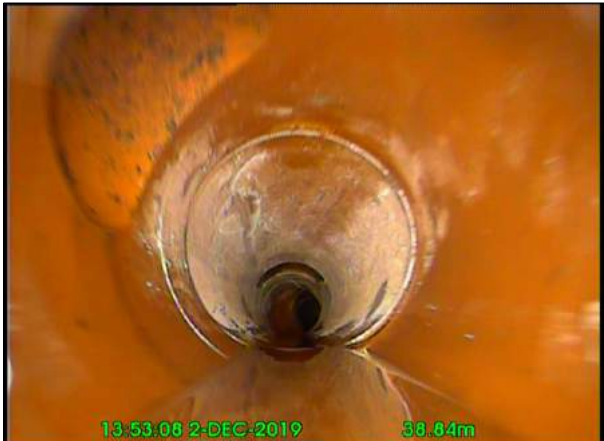
Photo: 24_18A 39.1m, Connection other than junction, at 10 o'clock, diameter 100mm
