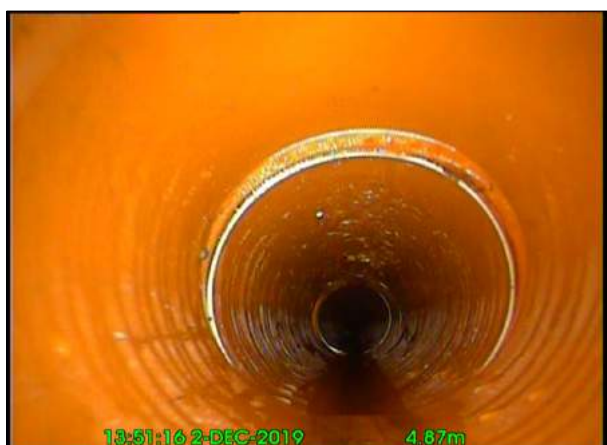
Photo: 24_4A 5.1m, Joint displaced, large
