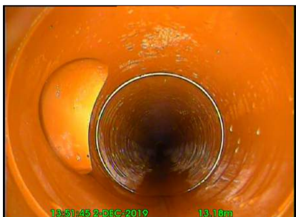
Photo: 24_8A 13.4m, Connection other than junction, at 9 o'clock, diameter 100mm
