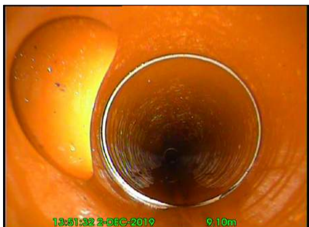
Photo: 24_6A 9.3m, Connection other than junction, at 9 o'clock, diameter 100mm
