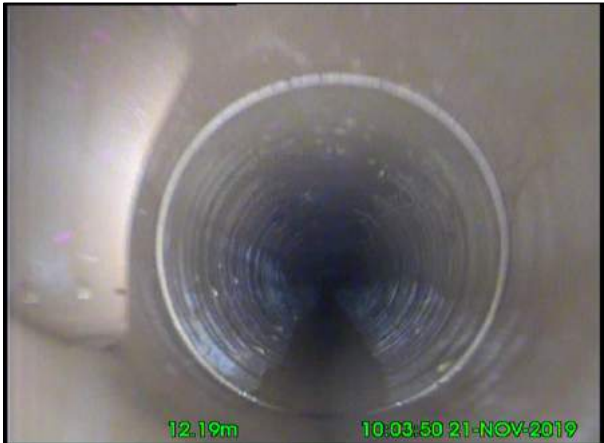
Photo: 15_7A 12.4m, Connection other than junction, at 9 o'clock, diameter 100mm
