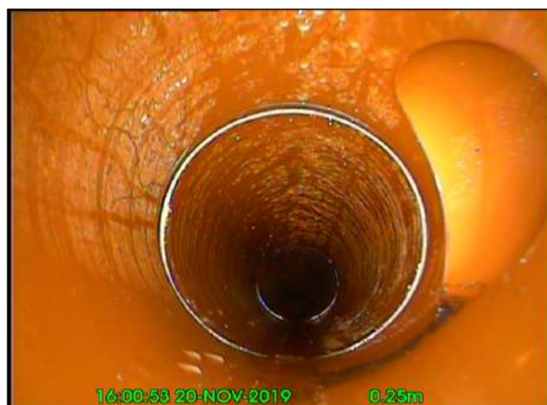
Photo: 9_3A 0.5m, Connection other than junction, at 3 o'clock, diameter 100mm
