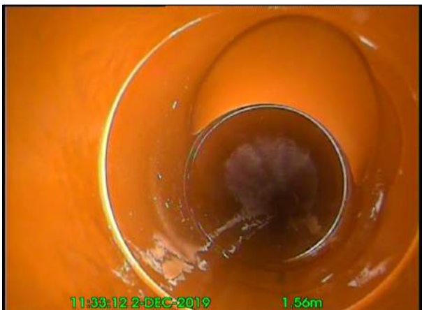
Photo: 22_4A 1.8m, Connection other than junction, at 12 o'clock, diameter 100mm
