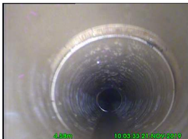
Photo: 15_4A 4.8m, Joint displaced, medium
