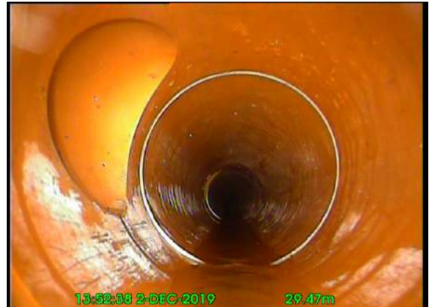
Photo: 24_15A 29.8m, Connection other than junction, at 10 o'clock, diameter 100mm
