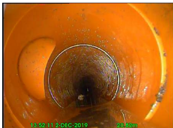
Photo: 24_11A 21.1m, Connection other than junction, at 9 o'clock, diameter 100mm
