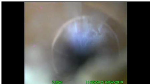
Photo: 13_6A 7.4m, Connection other than junction, at 1 o'clock, diameter 100mm
