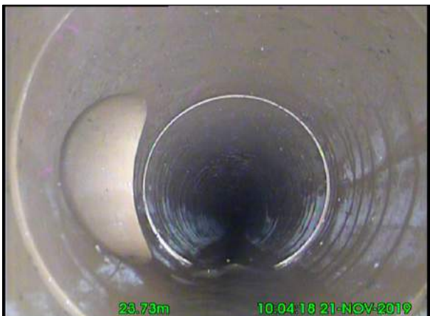
Photo: 15_14A 23.9m, Connection other than junction, at 9 o'clock, diameter 100mm
