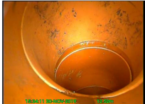
Photo: 6_9A 12.7m, Line deviates down
