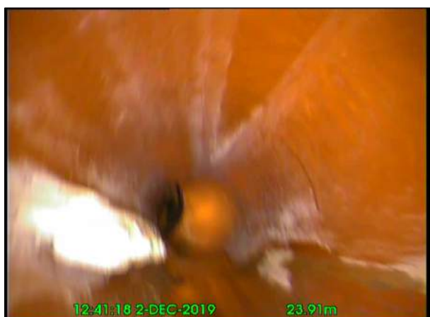
Photo: 20_12A 24m, Attached deposits, encrustation, from 8 to 9 o'clock, 10% cross-sectional area loss
