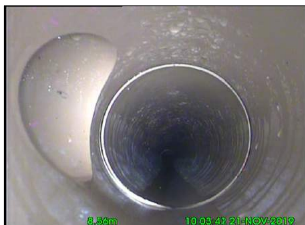
Photo: 15_6A 8.6m, Connection other than junction, at 9 o'clock, diameter 100mm
