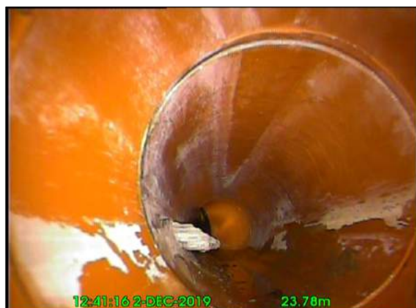
Photo: 20_11A 23.8m, Line deviates left
