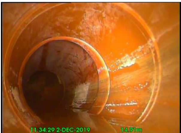
Photo: 22_8A 15.1m, Line deviates left
