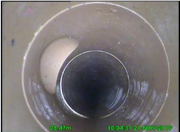
Photo: 15_16A 28.7m, Connection other than junction, at 10 o'clock, diameter 100mm
