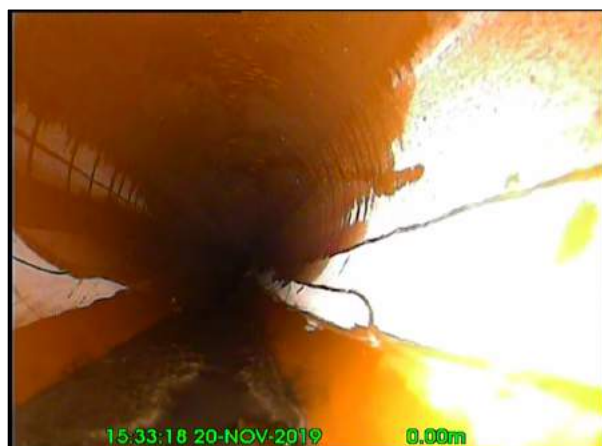
Photo: 6_3A 0m, Settled deposits, fine, 15% cross-sectional area loss, Start
