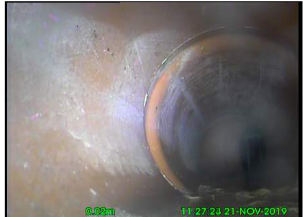
Photo: 18_3A 0m, Settled deposits, fine, 10% cross-sectional area loss, Start
