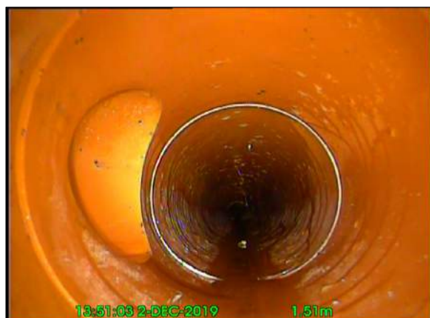
Photo: 24_3A 1.8m, Connection other than junction, at 9 o'clock, diameter 100mm
