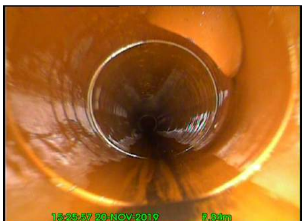
Photo: 4_4A 8.1m, Connection other than junction, at 1 o'clock, diameter 100mm
