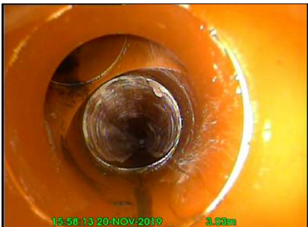
Photo: 10_4A 3.3m, Connection other than junction, at 11 o'clock, diameter 100mm
