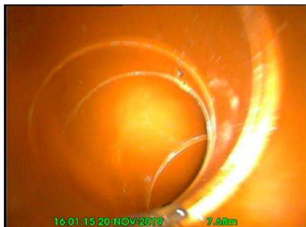
Photo: 9_5A 7.8m, Joint displaced, medium
