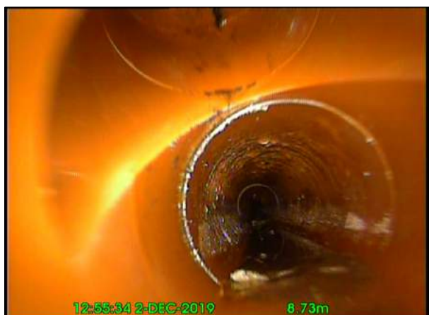
Photo: 21_6A 8.9m, Connection other than junction, at 11 o'clock, diameter 100mm
