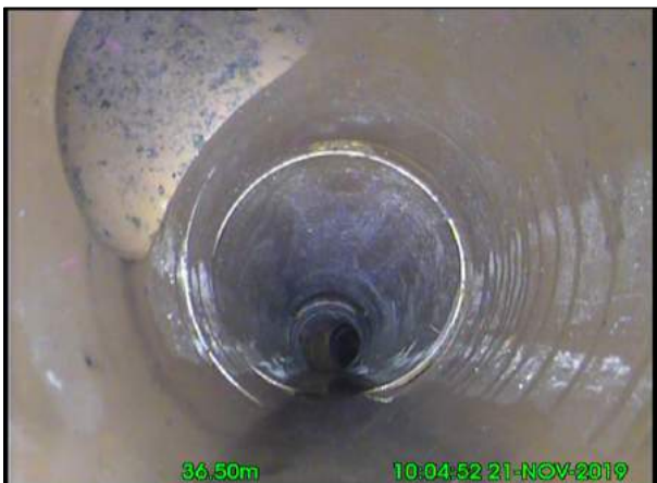
Photo: 15_18A 36.7m, Connection other than junction, at 10 o'clock, diameter 100mm
