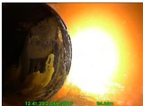
Photo: 20_13A 24.9m, Line deviates left
