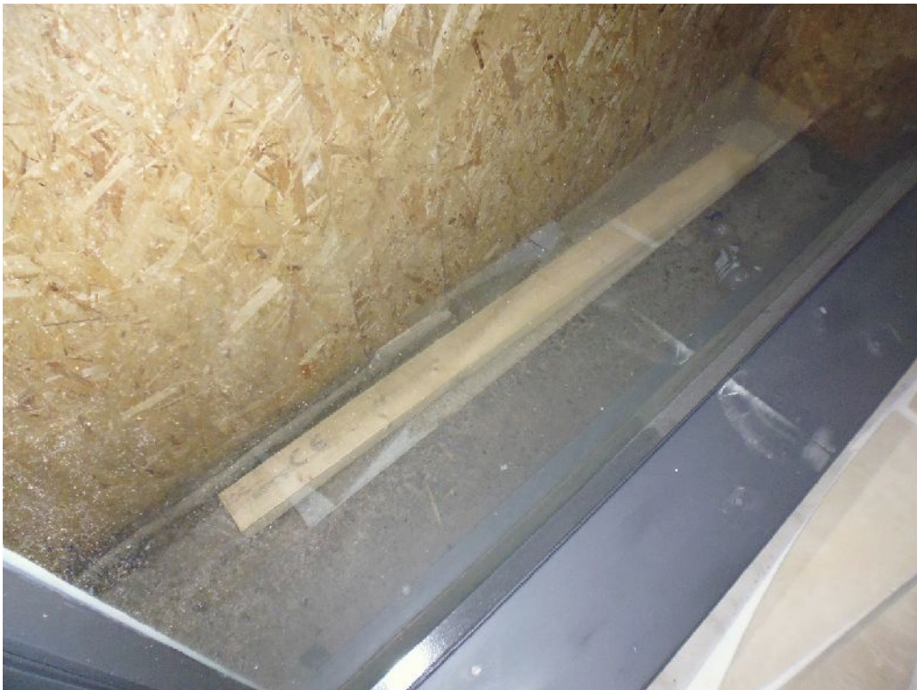
Pavement Light 6 - 2380mm x 500mm. Note the pavement light has been covered with concrete. The sizes are similar to Pavement Light 1.
