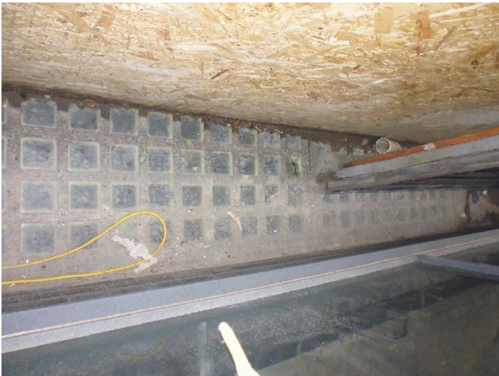
Pavement Light 4 - 2850mm x 600mm. Note the damaged glass blocks in various locations.
