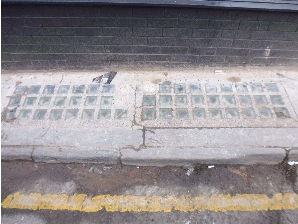
Pavement Light 1 - 2380mm x 500mm. Note the slight cracking to the concrete surround and some damaged glass blocks.
