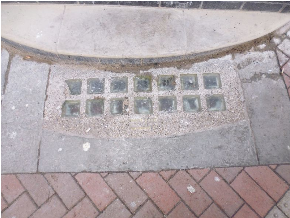
Pavement Light 2 - 1070mm x 400mm. Note the slight damage to the glass blocks.
