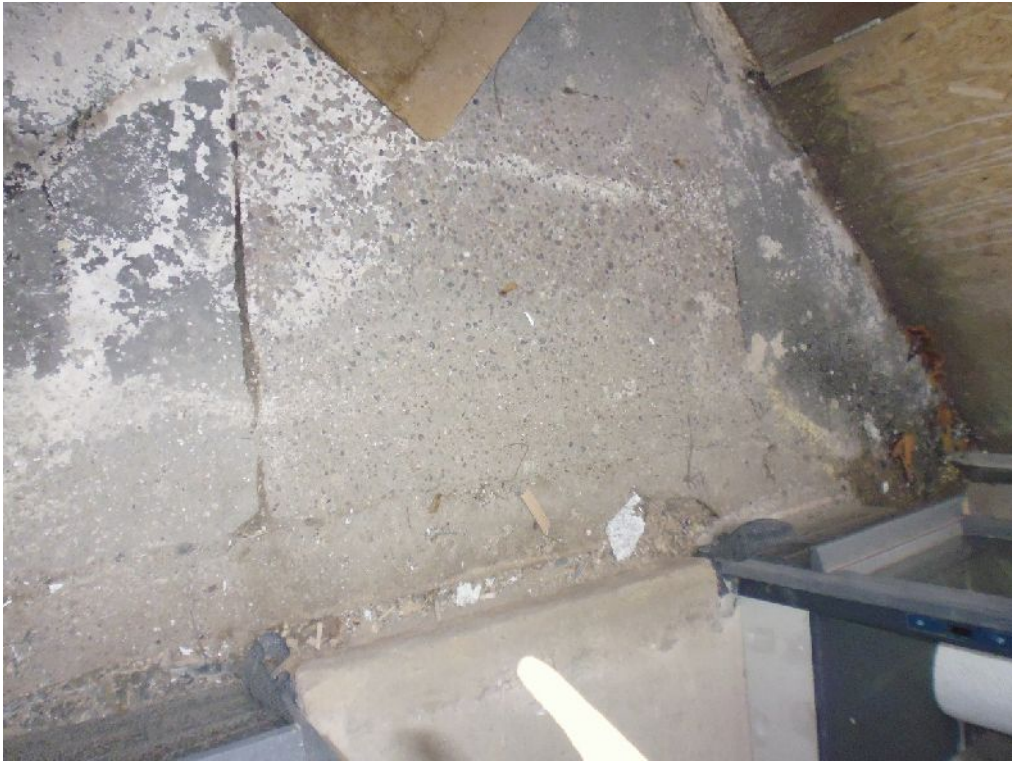
Pavement Light 5 - 1070mm x 400mm. Note the pavement light has been covered with concrete. The sizes etc. are similar to Pavement Light 2.
