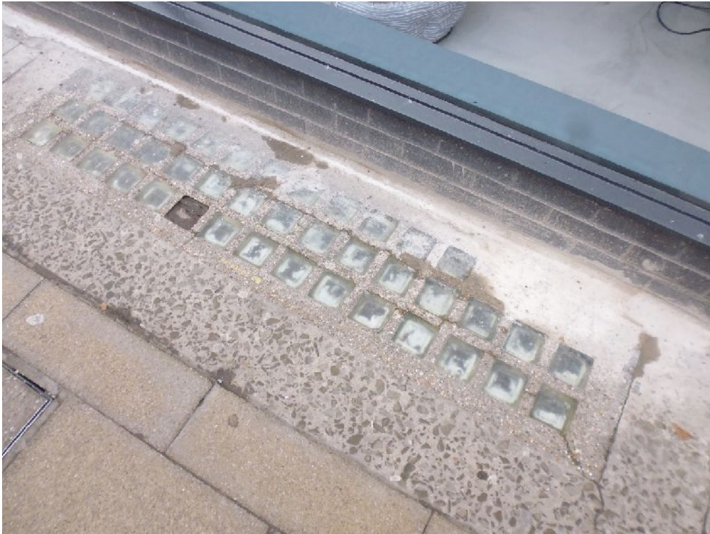
Pavement Light 3 - 2100mm x 500mm. Note the slight cracking to the concrete surround and some damaged glass blocks.
