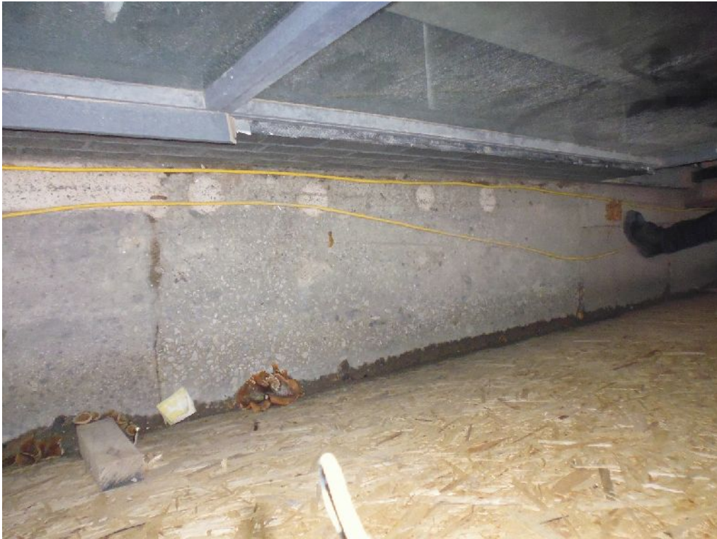
Pavement Light 7 - 1700mm x 600mm. Note the pavement light has been covered with concrete.
