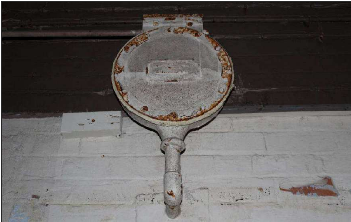
Plate 50: Sprinkler system fire alarm valve, Ground floor
