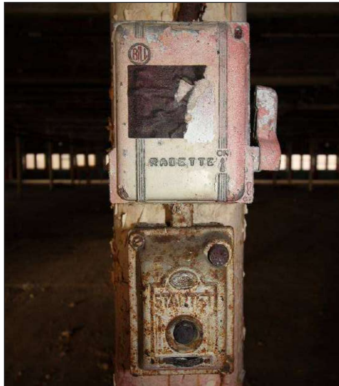
Plate 84: Detail of the electrical switch boxes mounted on a third-floor column
