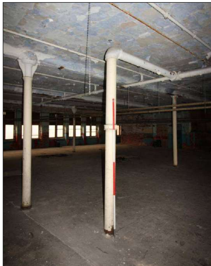
Plate 85: Top of vertical pipe of sprinkler system jointed into diminishing pipes of the upper floor
