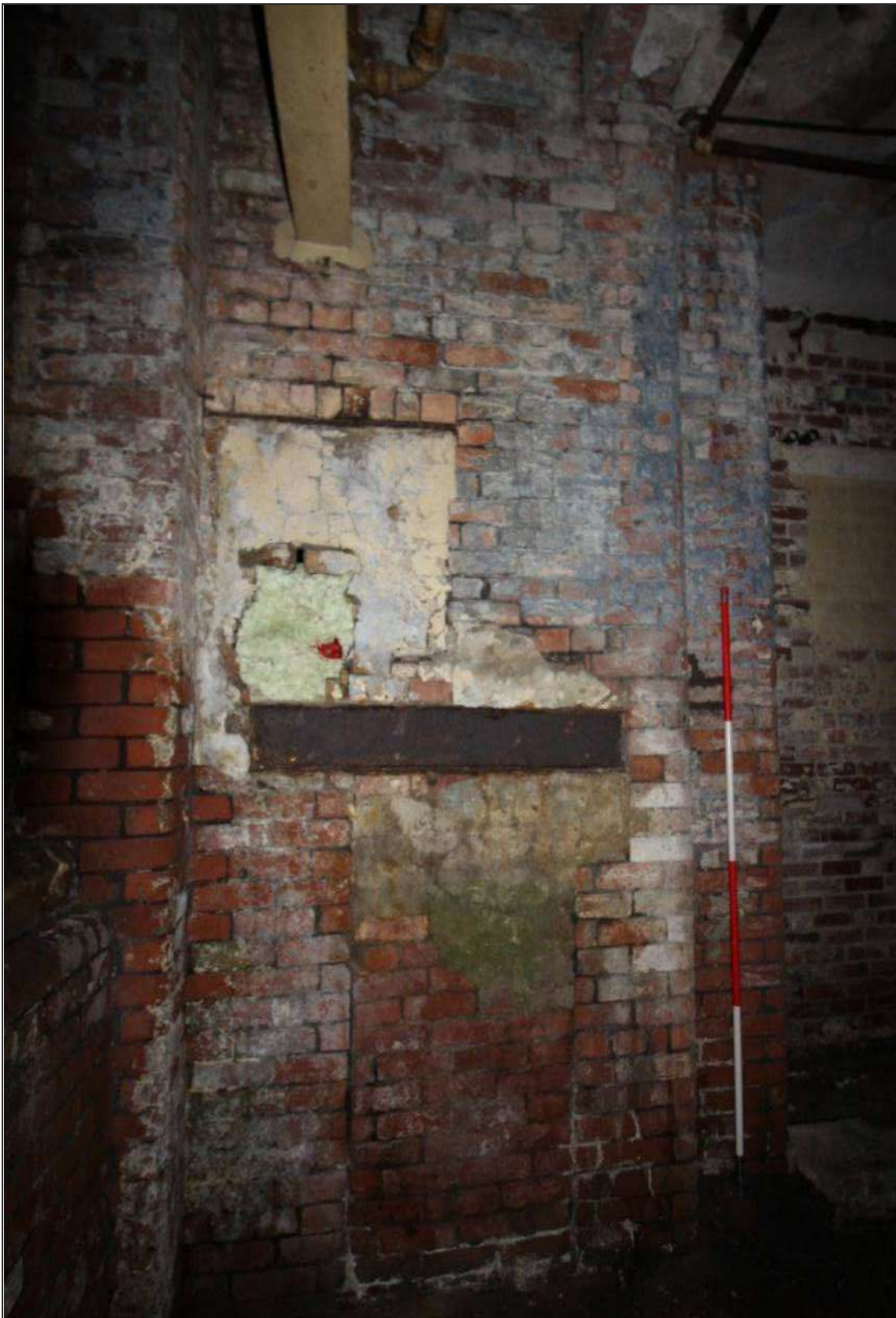
Plate 57: Two blocked flues leading into the chimney
