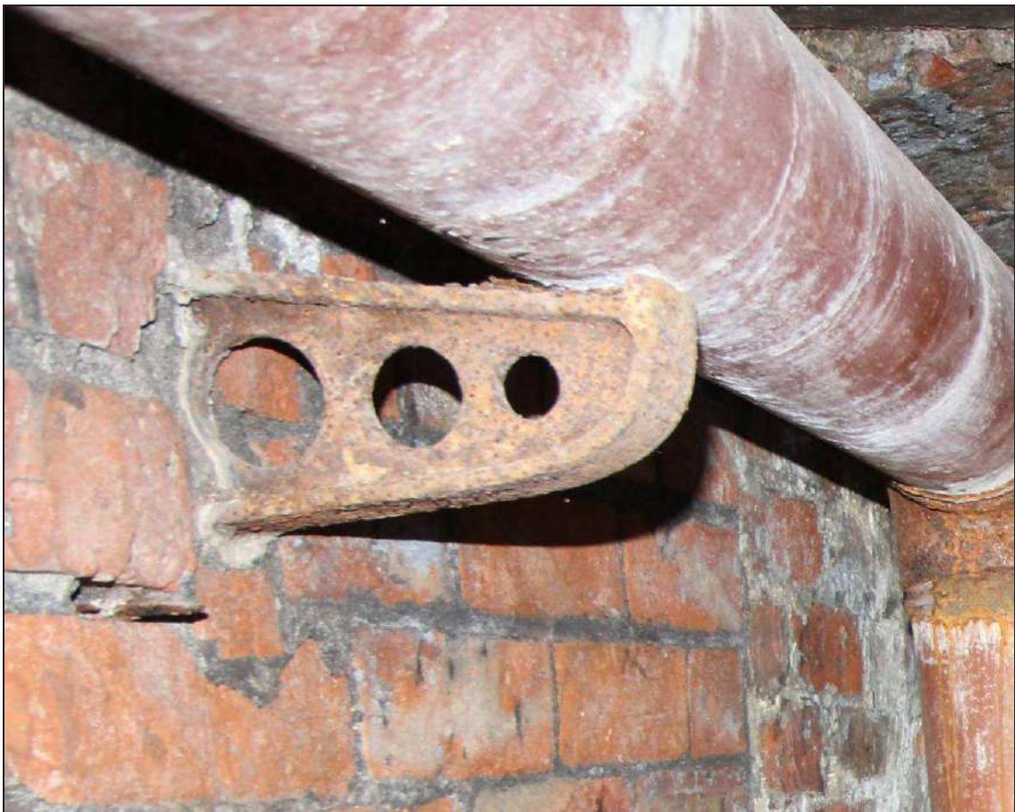
Plate 46: Detail of the brackets supporting the pipework within the tunnel
