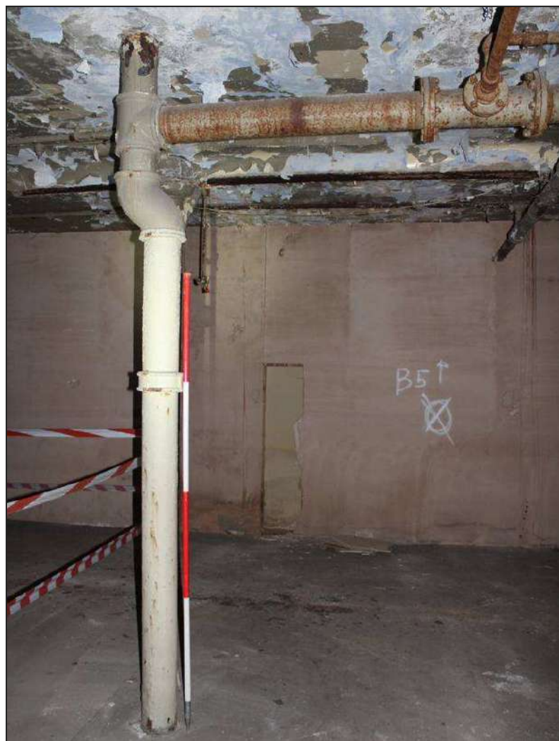
Plate 49: Vertical pipe at ground-floor level transferring water between floors for the sprinklers
