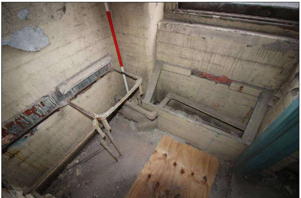
Plate 81: Washbasin stands and shuttered pipework, second floor
