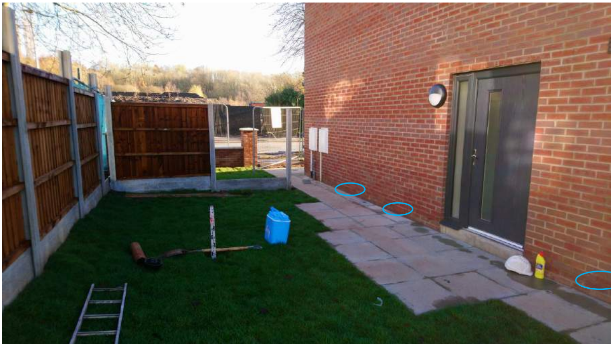
Photograph 12 Plot 10 showing pit location. The locations of the external sub-slab vents are also indicated in blue.
