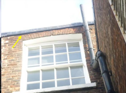
P4 Gap under fascia, to rear
