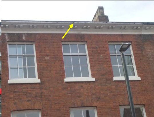
P2 Gap in eaves next to street lamp
