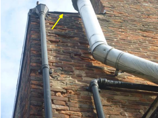
P5 Gap under end slate to rear
