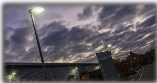
(Thorlux Starbeam LED as installed)
