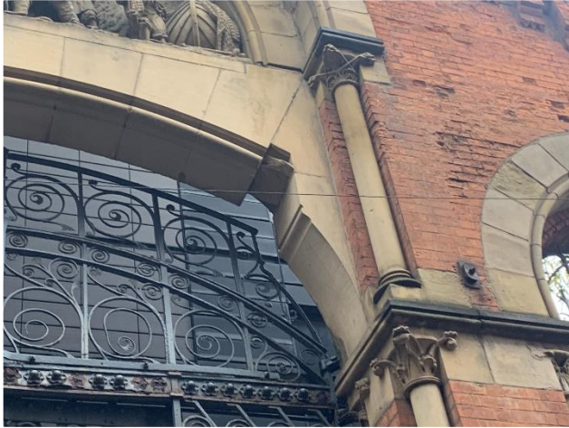
Damaged stone and dropped stone to arch.
