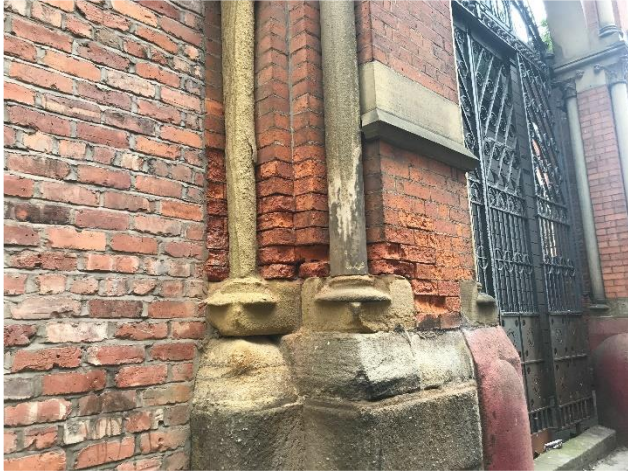
Spalled masonry and worn stone column.
