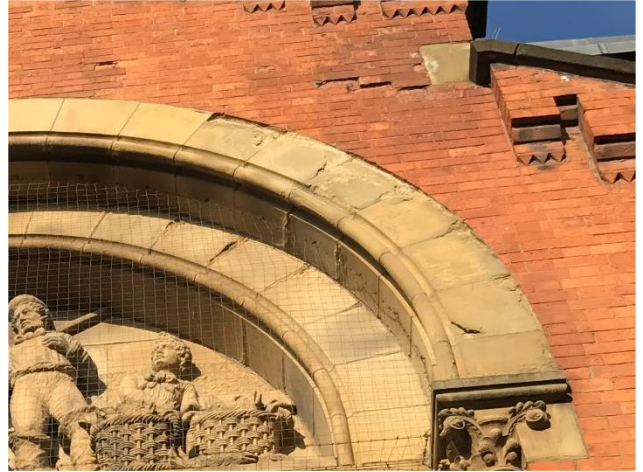
Worn stonework to arches.
