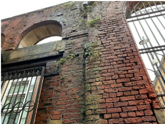
Vegetation and open joints.
