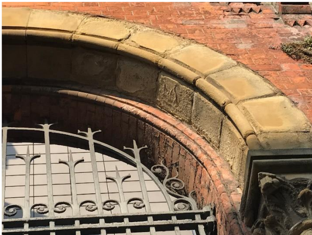
Worn/blistered face to stone arches.
