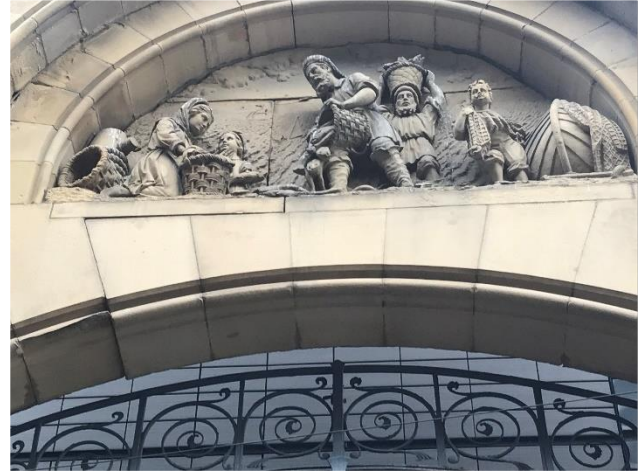
Arch – slipped stonework.
