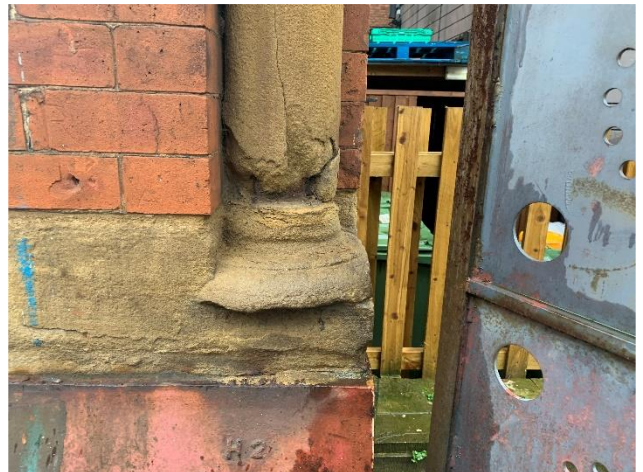
Corroded stone column.
