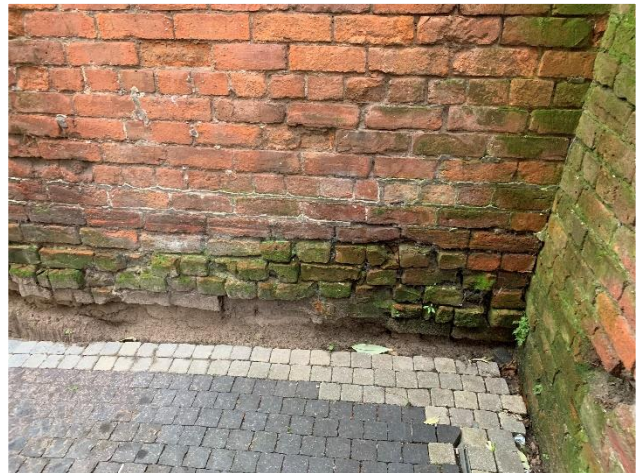
Corroded masonry and open joints.
