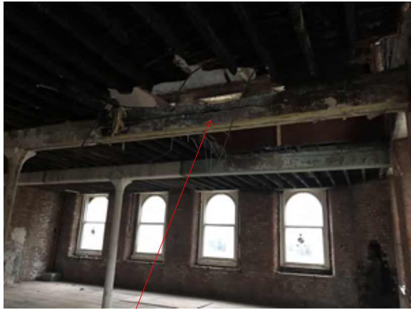
DAMAGED TIMBER TO BE REMOVED AND PACKED
