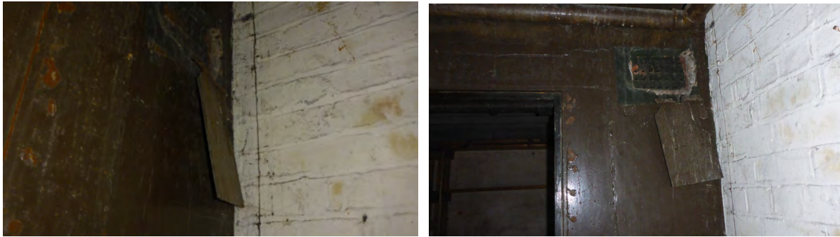
Small asbestos cement board panel to the Safe Room air vent
