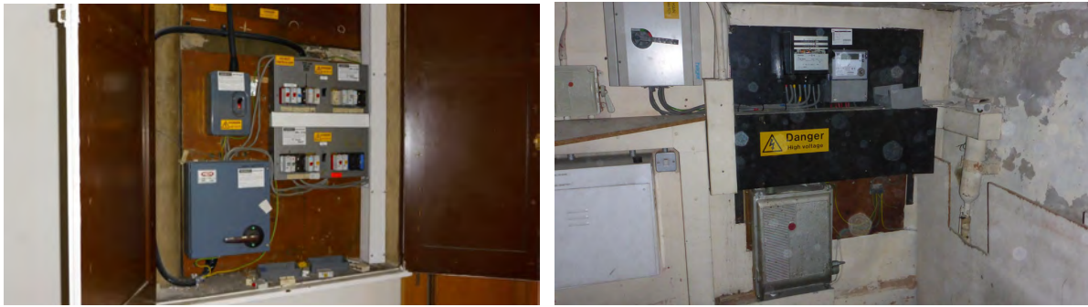
Internal asbestos components to old electrics throughout the building
