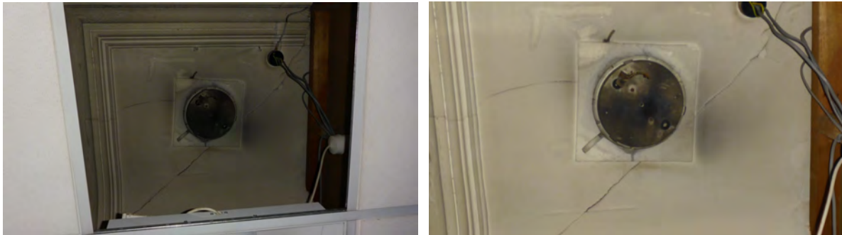
Asbestos insulation board panel to the original Half-landing ceiling between the first and second floor
