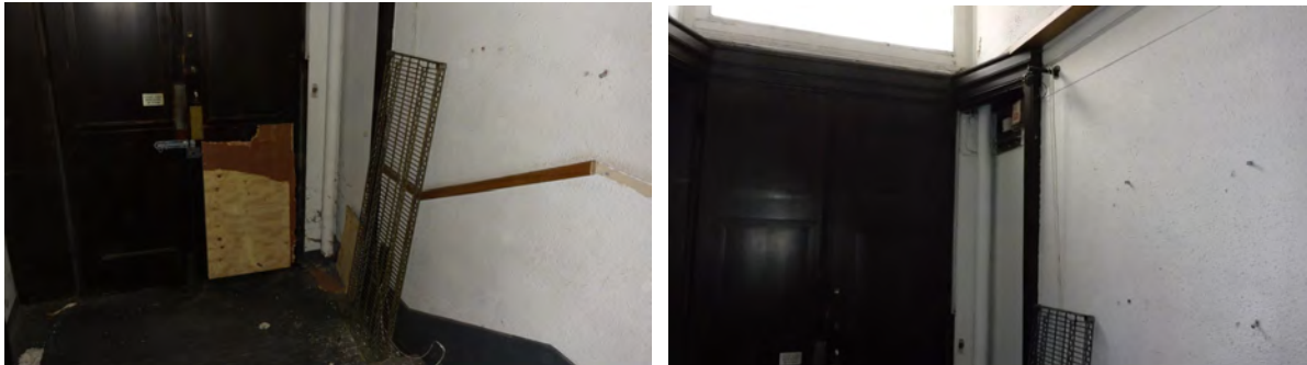
Asbestos thermal insulation to the vertical pipe beside the door
