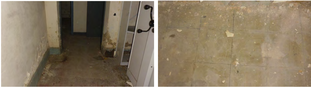
Asbestos tiles to the File Store and Lobby floors
