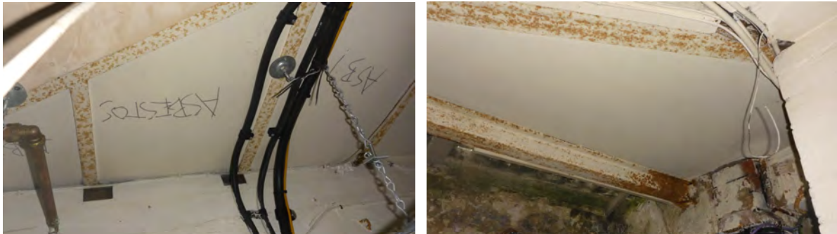
Asbestos cement boarding to part of the ceilings
