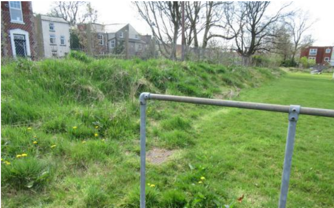
Junior grass pitch drain chamber - running to the main chamber in the distant corner
