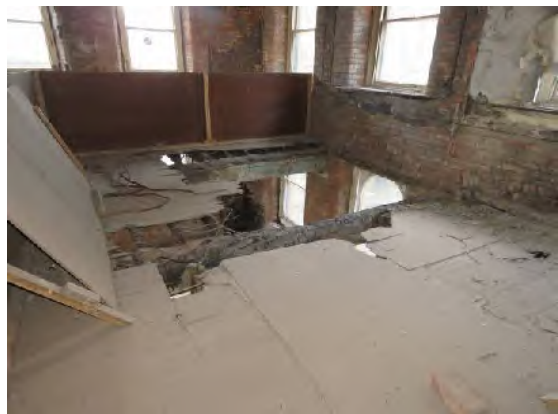
Figure 27: photo of the damage caused by the 2012 fire to the floor.
