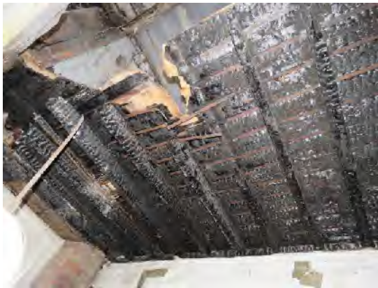
Figure 23: photo illustrating the damage to the ceiling caused by a fire in 2012
