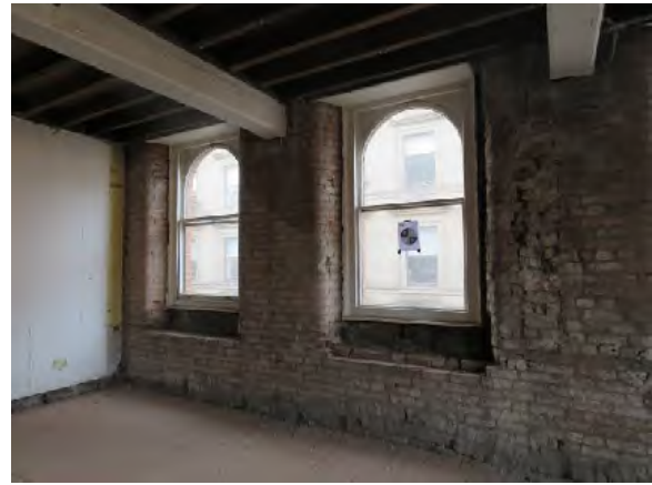
Figure 22: detailed view of the typical condition of the windows illustrating loss of internal dressings/ sills and wall coverings.
