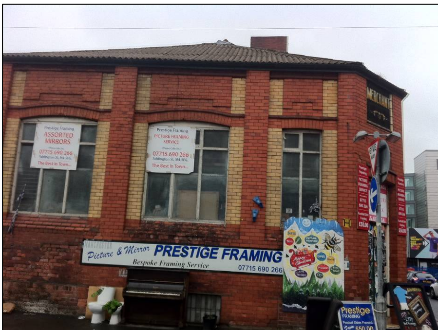
Plate 2 Exterior elevation, facing onto Chadderton Street, showing asbestos roof
