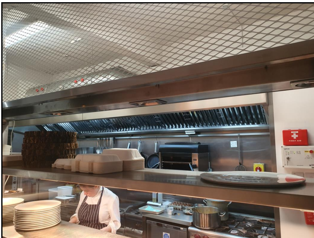
Fig 6 – Photo showing the restricted height and space for the required internal ESP followed by carbon filtration system that was required.
