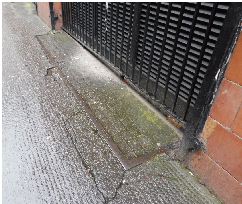
Existing pavement lights currently blocked
