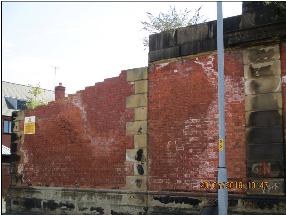
Plate 3 Degraded brickwork on external corner of Cross Keys Street and Bendix Street
