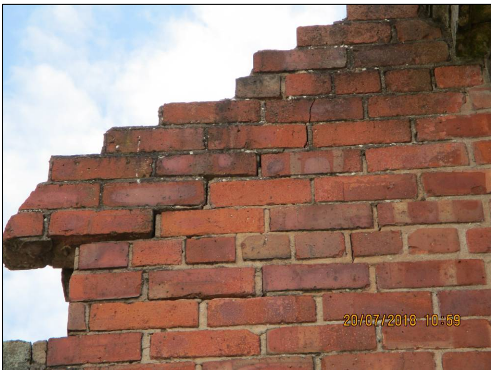
Plate 4 Close up of crevice within degraded brickwork
