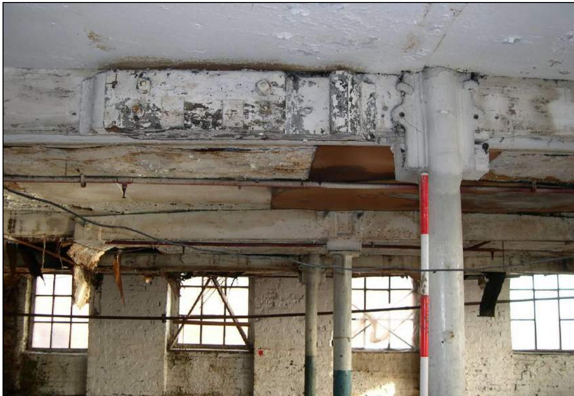
Plate 21: Sole plate to house the vertical transmission on the fourth floor of Decker Mill
