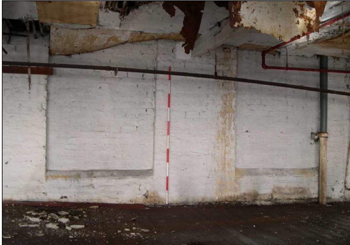
Plate 22: Blocked windows in the north elevation on the forth floor of Decker Mill
