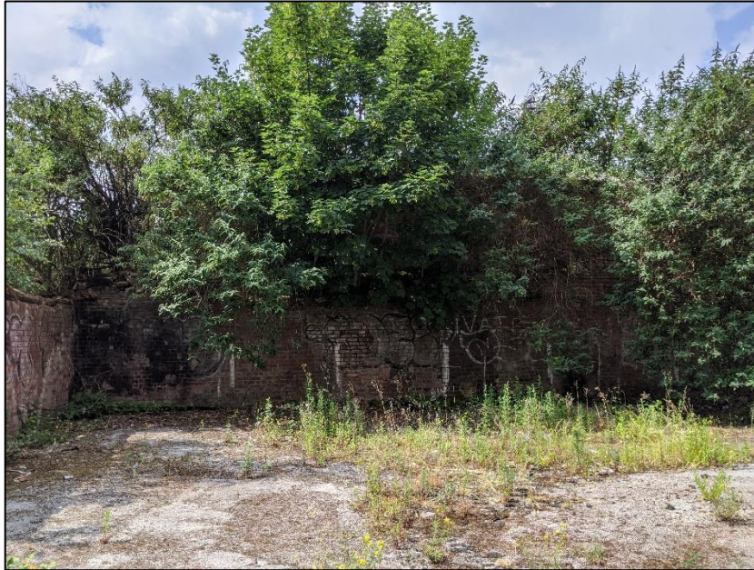
Photograph 7 showing the overgrown vegetation
