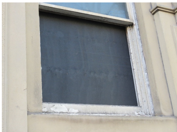
17. Example of flaking paint to window frame and sash.
