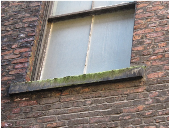
25. Example of moss growth to window cill.
