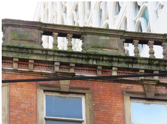
3. Example of algae growth and salt efflorescence to parapet.
