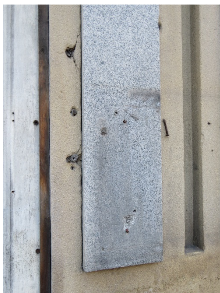
9. Example of scarring to façade from earlier fixings.
