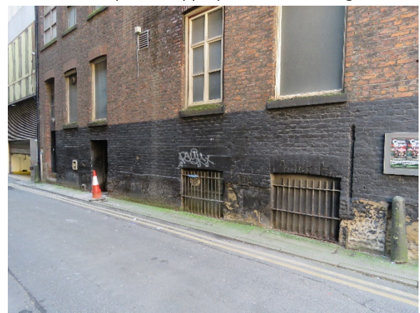
24. The application of masonry paint and erosion of sandstone at ground level.
