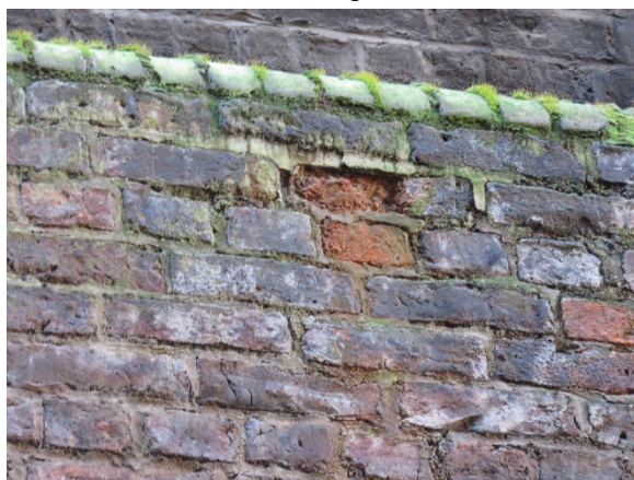
23. Example of erosion to brickwork and cement pointing.
