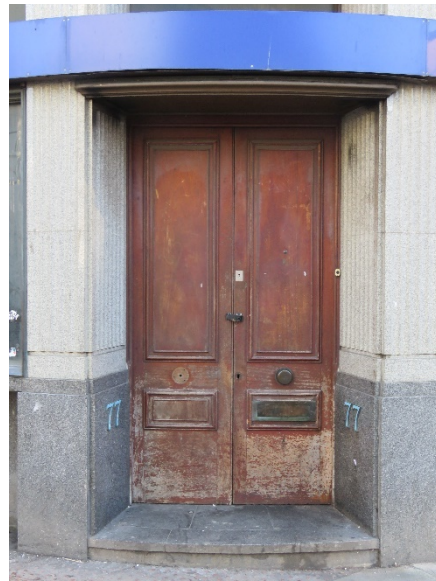
20. Example of wear and damage to the timber doors.
