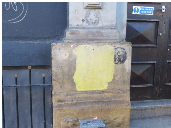
15. Example of paint to sandstone.
