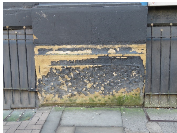
16. Example of masonry paint and eroding sandstone to the ground floor with modern rails either side.
