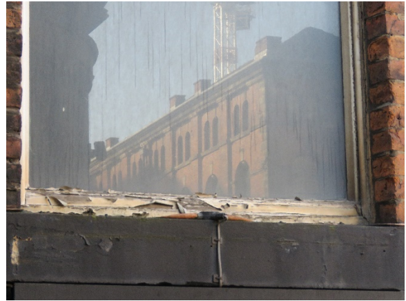
26. Example of failing paint system to window.
