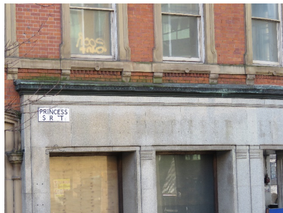
14. Example of staining to granite cladding.
