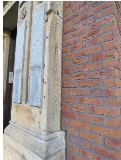
2. Example of damaged sandstone.
