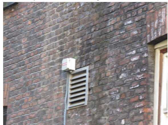
22. Example of inappropriate ventilation grill.
