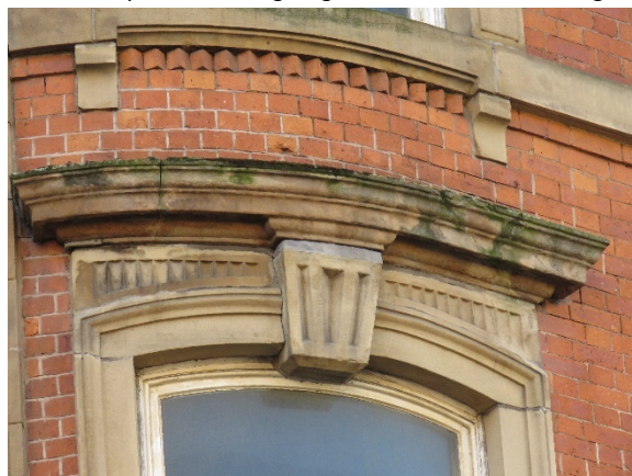
12. Example of algae / moss growth to sandstone window head and erosion of stone.
