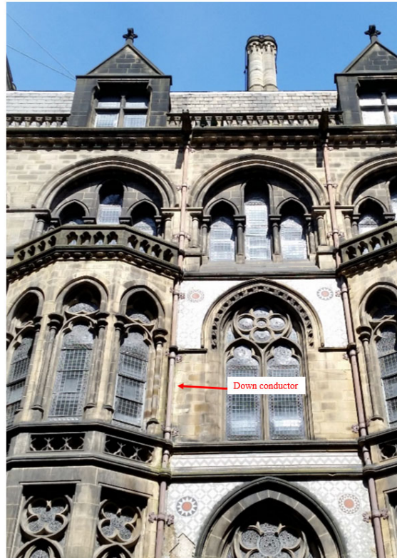
Figure 3 – Existing copper wire down conductor
