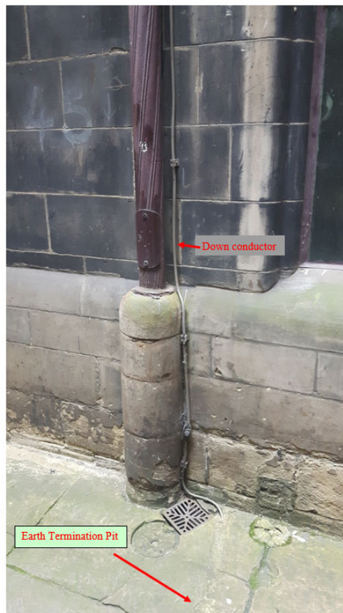
Figure 4 – Existing copper wire down conductor connecting into the below ground earth terminal
