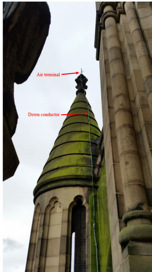
Figure 1 – Existing copper multi point air terminal rod connected to a copper down conductor
