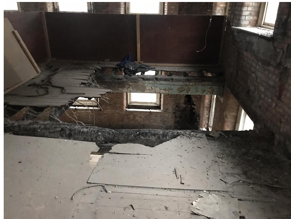
Figure 2.2: Photograph of Fire Damaged Floor at Third Floor
