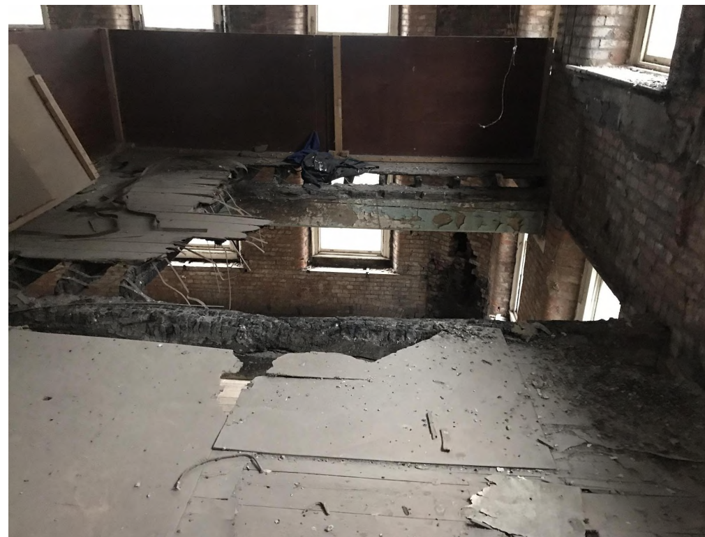
Figure 2.2: Photograph of Fire Damaged Floor at Third Floor
