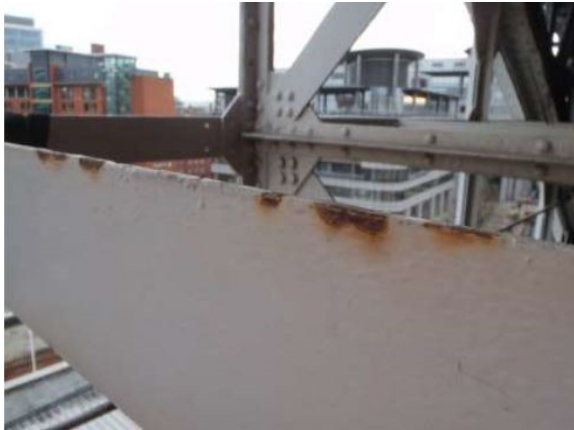
Coating removed by mechanical damage
