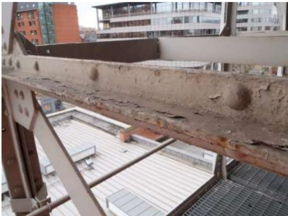
Flaking and delamination of the top coat
