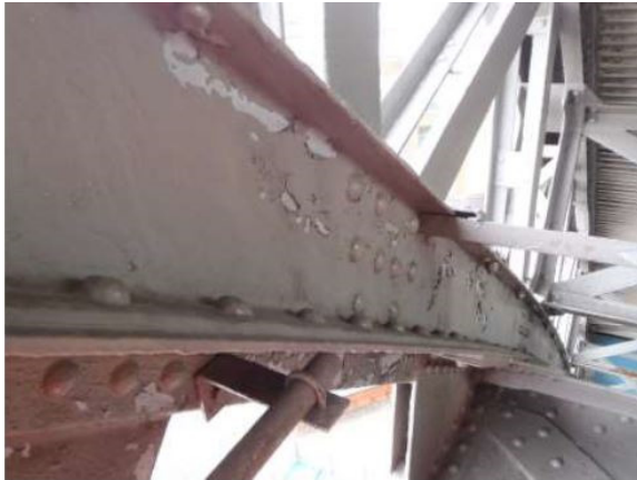
Flaking and delamination of the top coat
