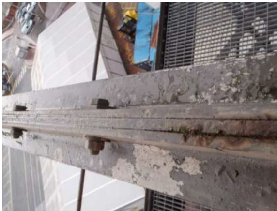
Rust staining in the back to back gaps filled
