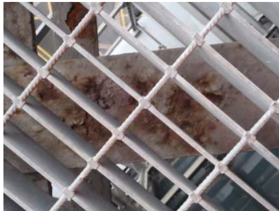
Corrosion under the walkway grating
