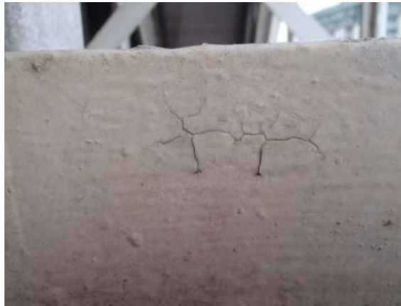
Cracking of the coatings
