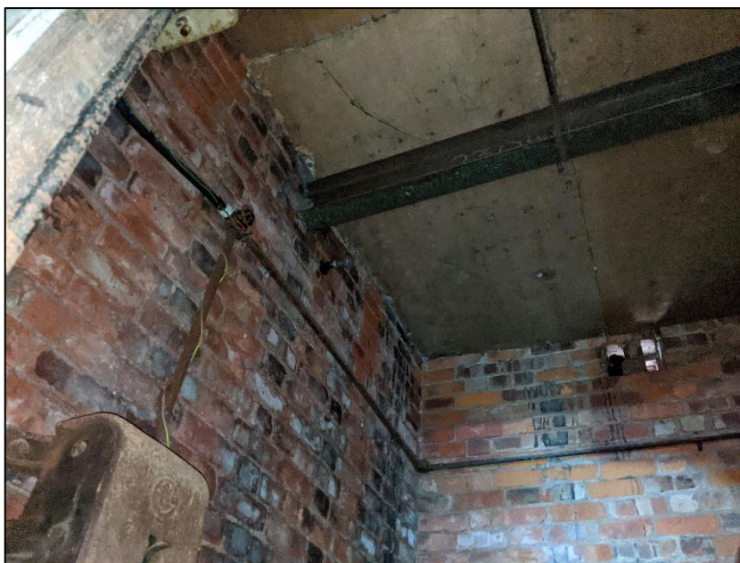
Photograph 5 showing the lift motor room
