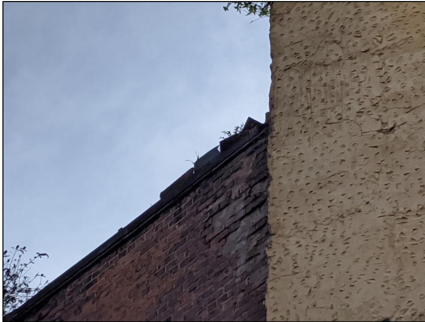
Photograph 2 showing the broken roofing tiles
