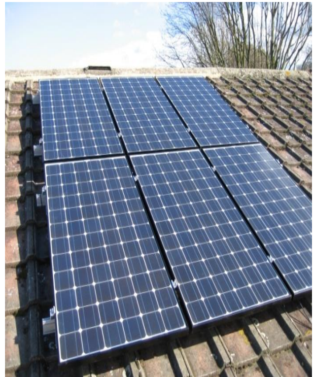
Figure 5 - Photovoltaic array on a pitched roof
