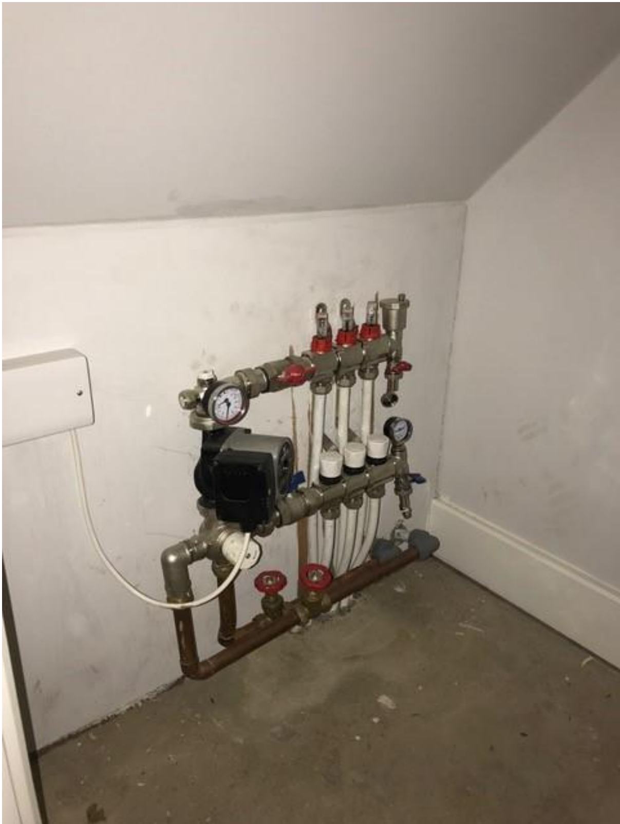
Insert 6: Central Heating – Under Floor Heating Manifolds
