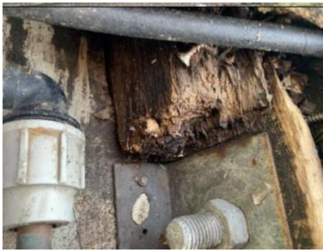
Supporting Joist End Completely Rotted
