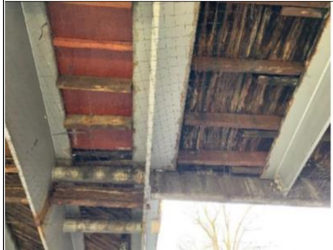
Walkway and Bridge from Below – Floorboards Completely Rotted and Joists Inadequate
