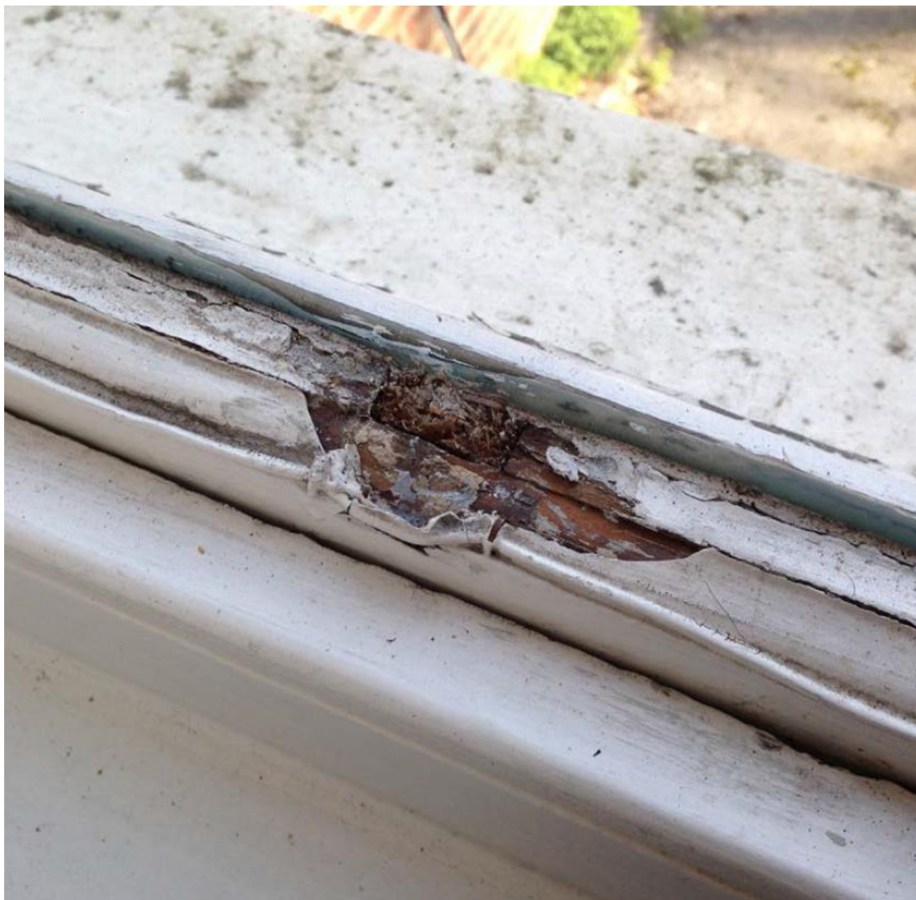
Plate 9: Damaged Window Frame, provided by Orco Heritage Statement 2014 (revised 2016)
