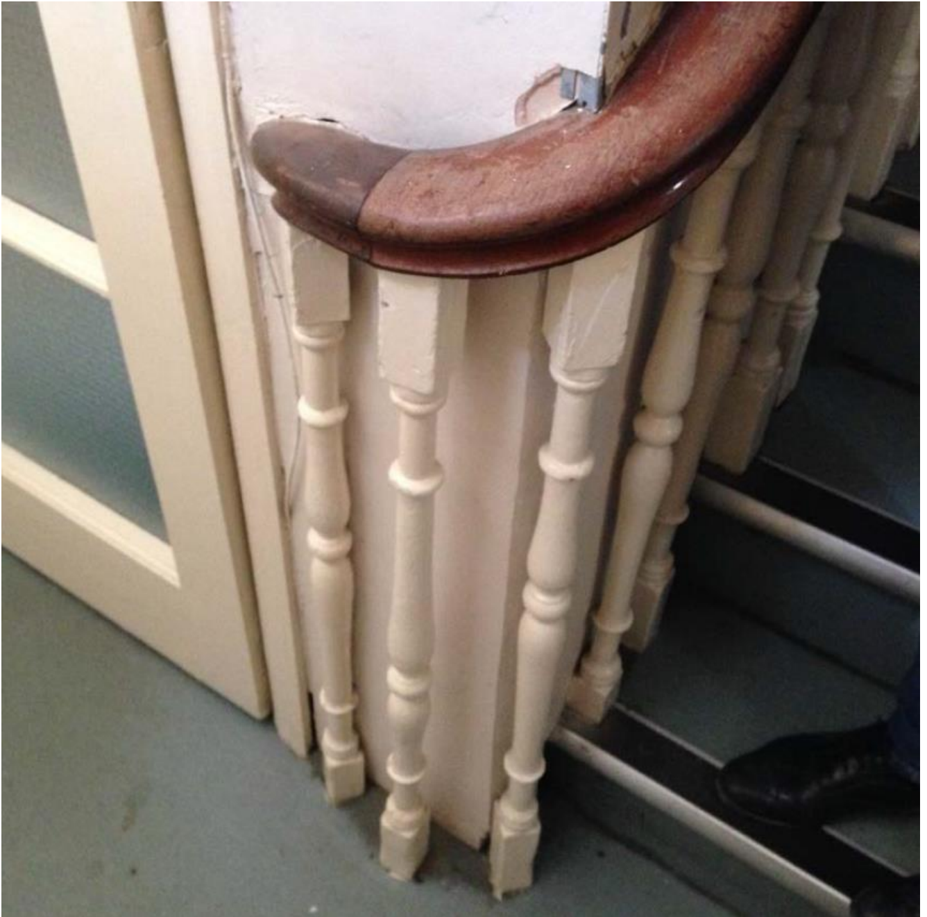
Plate 11: Staircase Door and Partition, provided by Orco Heritage Statement 2014 (revised 2016), showing poor quality 20 th century alterations
