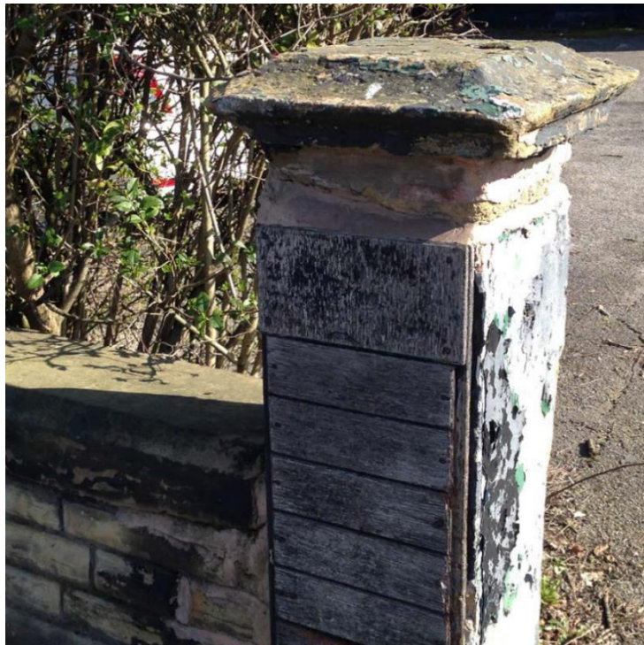
Damaged Pier, provided by Orco Heritage Statement 2014 (revised 2016)
