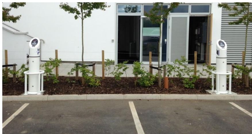
Fig 3.4 – Floor mounted post concrete plinth on soft ground - plinth dimensions are 0.6mx0.6mx0.6m
