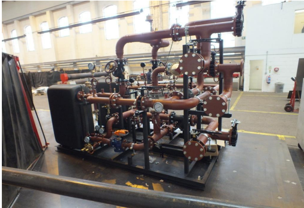
Figure 22 - Typical heat-substation. (Uninsulated).
