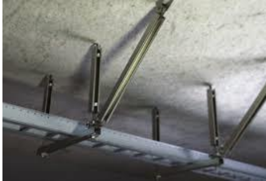
Figure 23 - Example Cable Ladder
