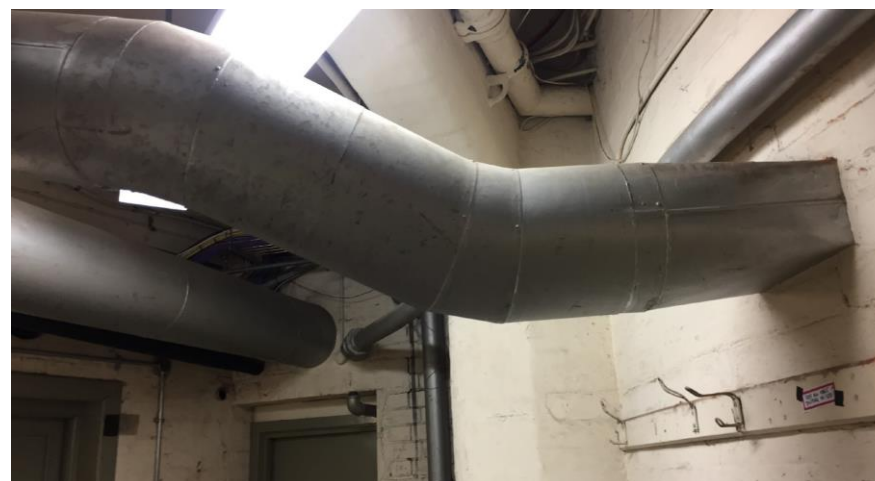
Figure 4 The air filtration equipment (proposed for removal and partially retained in LG)
