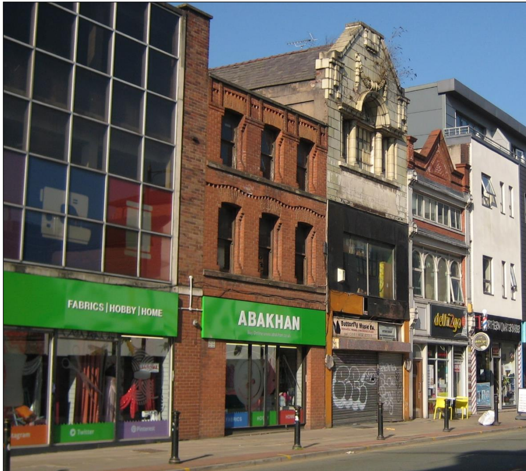
Figure 9: Poor quality signage/shopfronts and condition of buildings.
