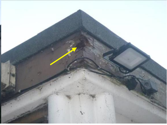
P6 Rot hole, boiler house
