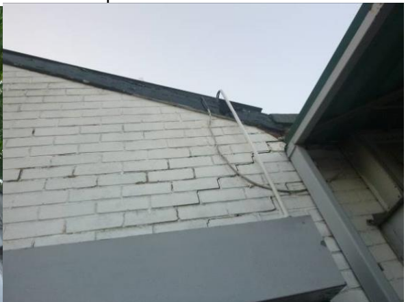
P4 Gap in masonry
