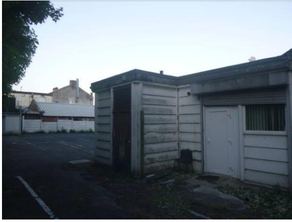
P5 Boiler house
