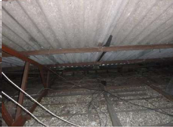
P8 Loft showing daylight at eaves
