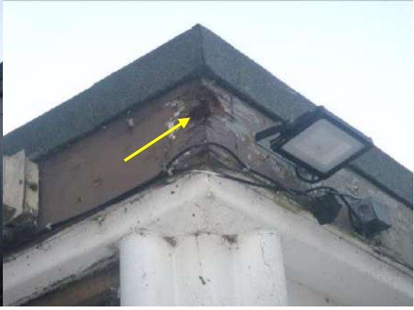
P6 Rot hole, boiler house
