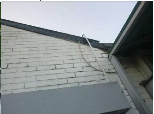
P4 Gap in masonry
