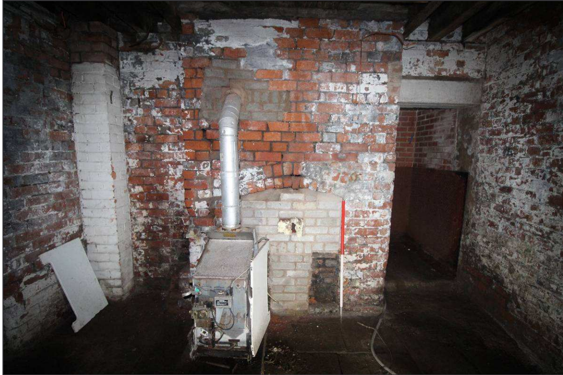
Plate 77: The modern boiler with the blocked-up fireplace behind
