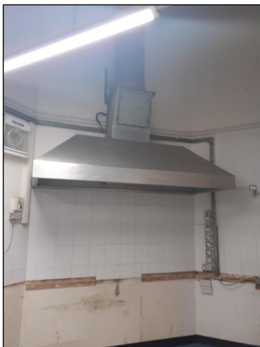
Figure 8: View of existing cooker hood to be reused.
