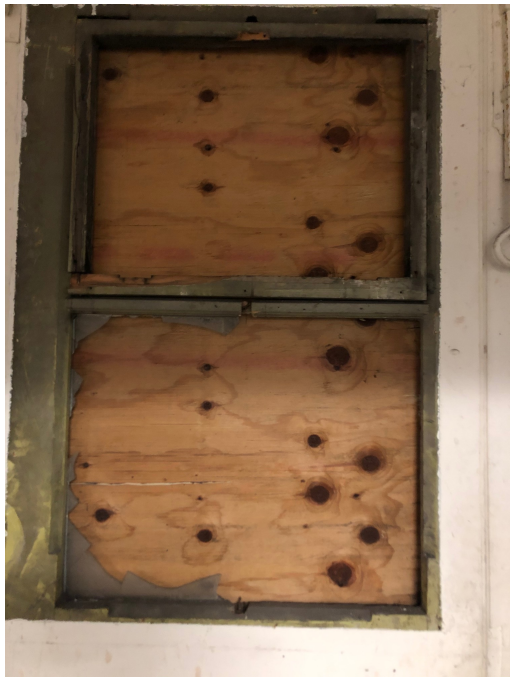
Existing glazed panels missing or broken.
