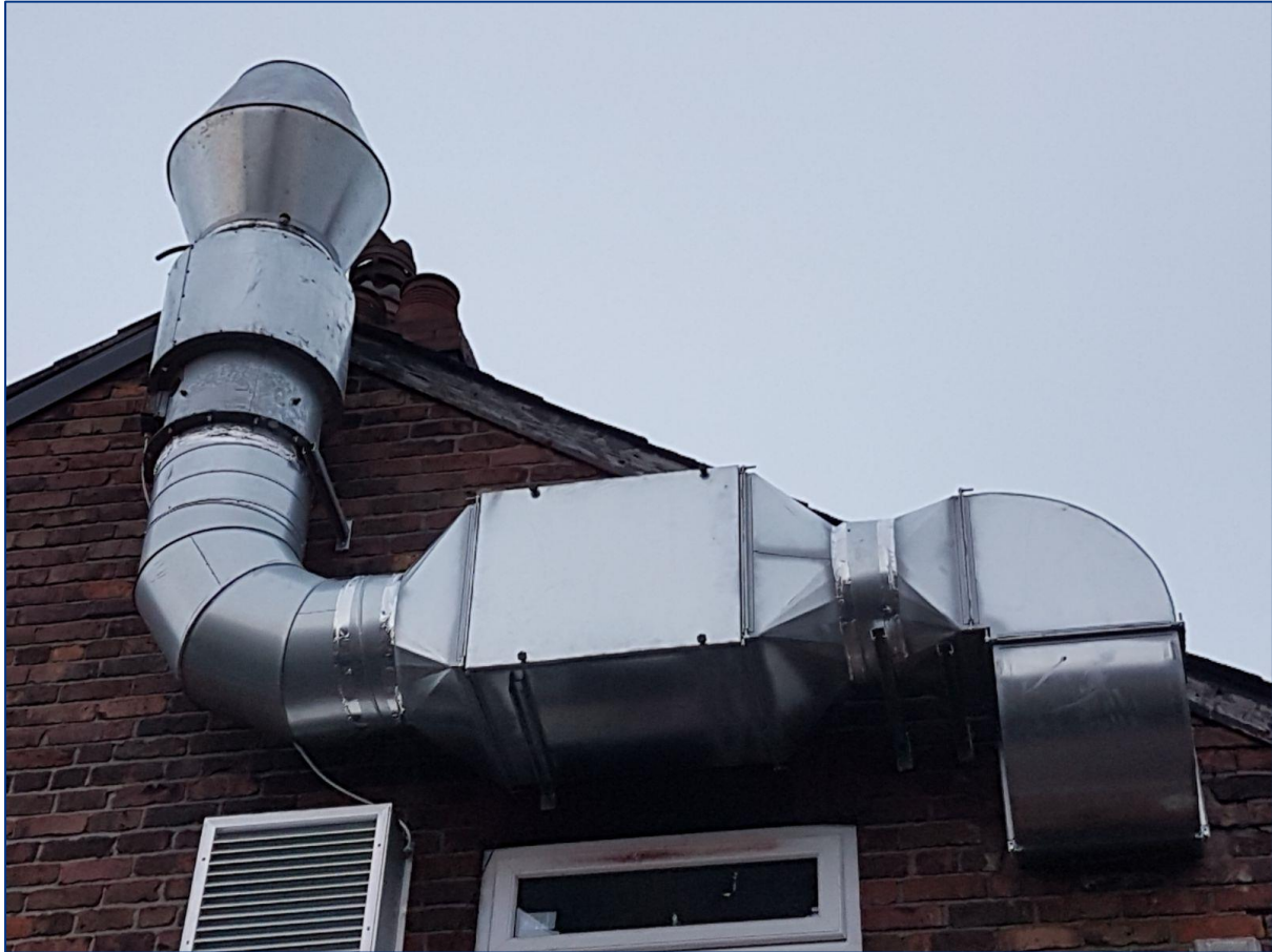
Figure 1: Installed Kitchen Extract
