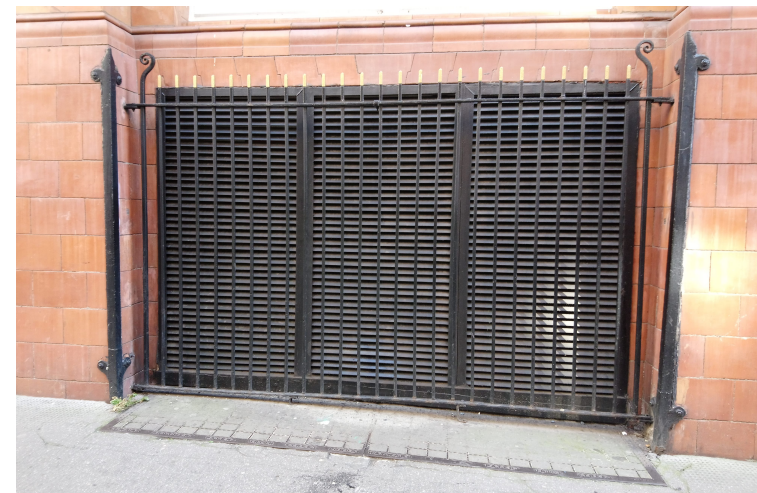
Photo of existing louvred window with cast iron railing on Great Bridgewater Street - glazing to be reinstated to 4no. windows
