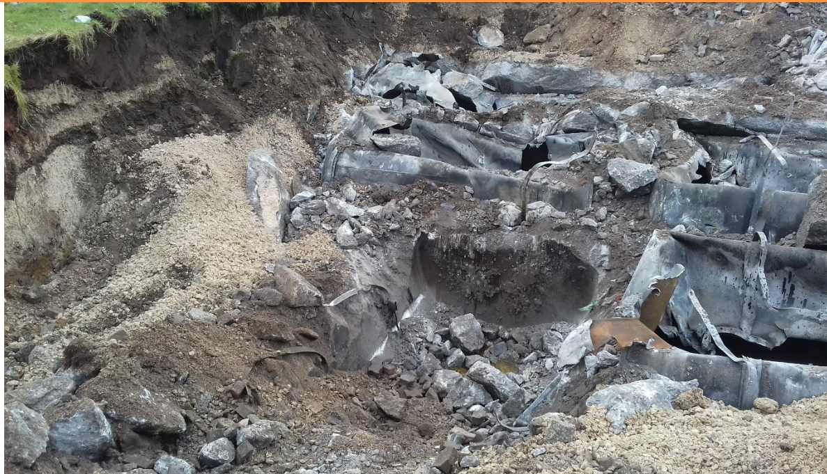
PLATE 10 – SUSPECTED FUEL IN CONCRETE CASING BENEATH TANK 1
