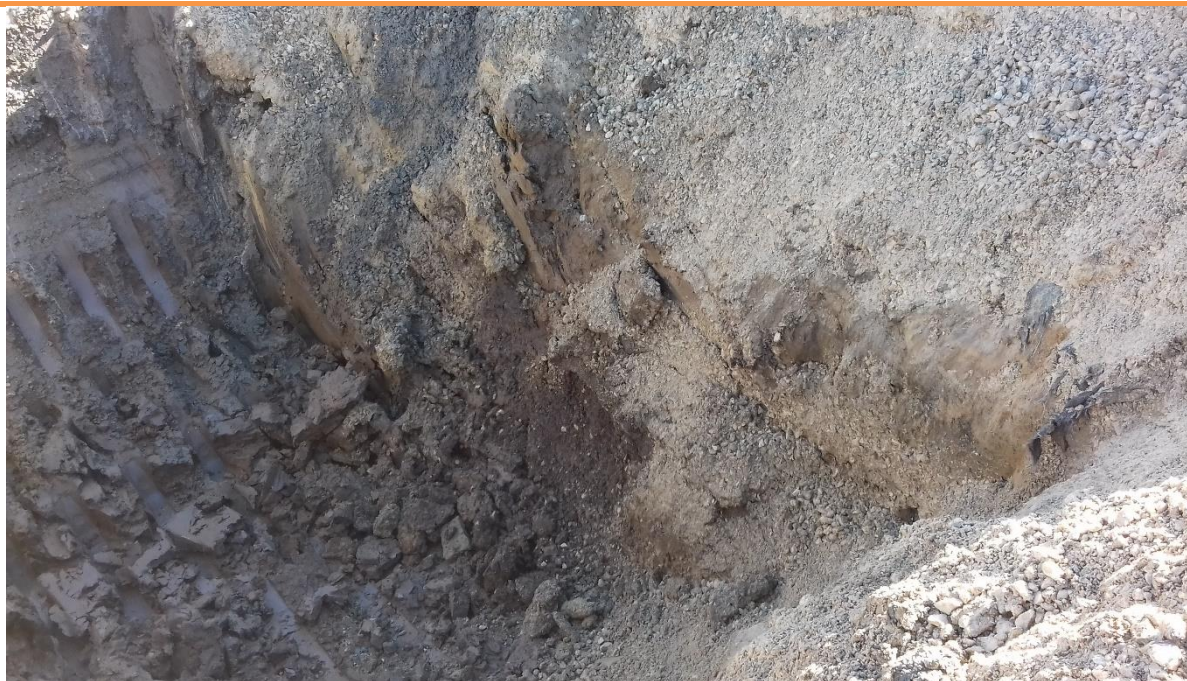
PLATE 19 – RESULTING VOID FOLLOWING REMOVAL OF INTERCEPTOR
