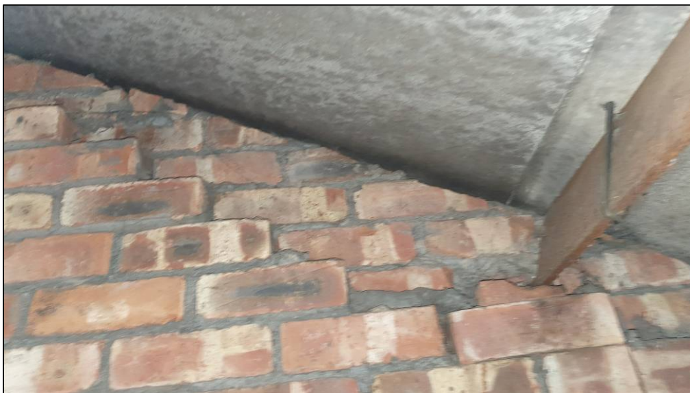
Plate 7 Gaps between asbestos roof and top bricks
