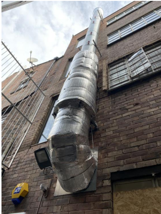
Figure 1 – Kitchen Extract Fan and Ductwork
